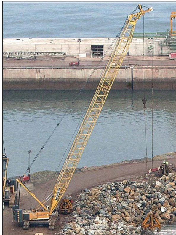
Figure 8 – Example of armour placement using orange peel grab carried out by Dragados
