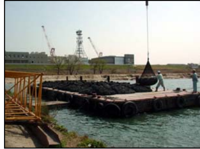
④ Load Filter Unit on a pontoon and bring them to installation area.
