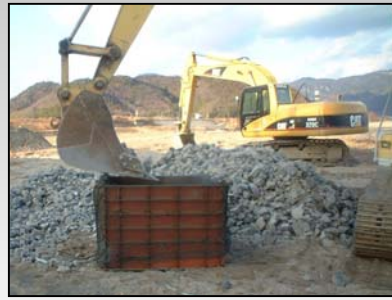
① Set Filter Unit in a production frame. Stuff stones by an excavator.
