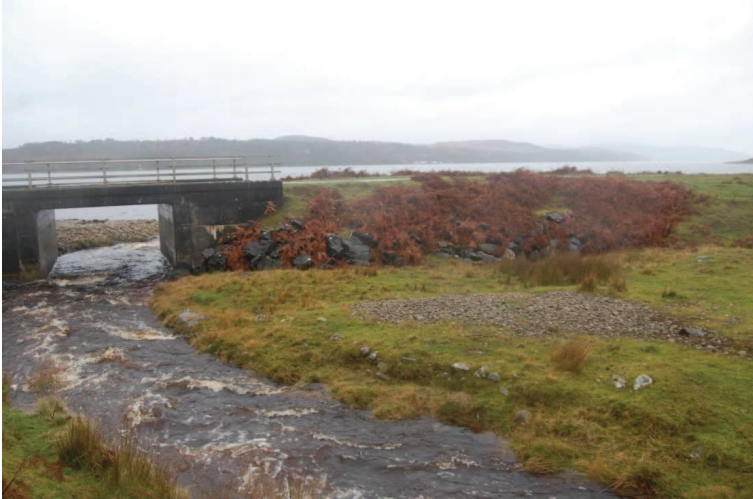
Plate 4.2 Rock armouring around the road bridge (all four sides) over Abhain Mhor – potential otter lie-up site (Survey Site B).
