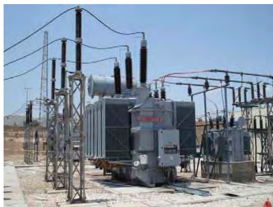
Figure 4.14 Example outdoor 33kV substation
