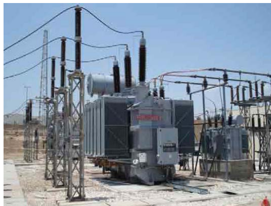
Figure 4.14 Example outdoor 33kV substation
