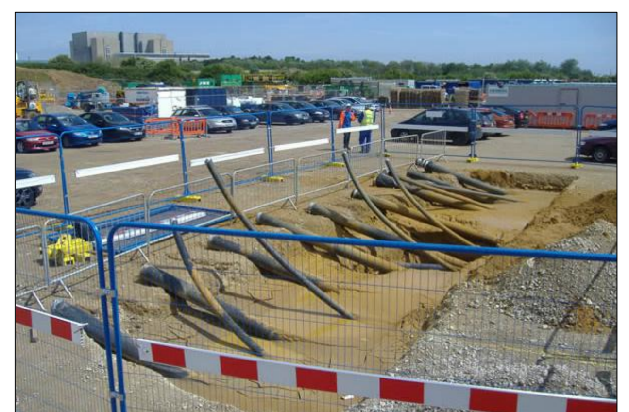
↑ Power cables installed at the Greater Gabbard offshore wind farm by HDD
