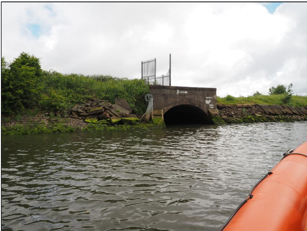
Photograph 2: Main Crossing North Pier Location at Existing Yoker Burn Culvert Outlet Position
