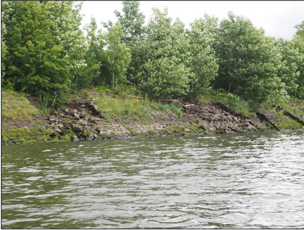
Photograph 5: Existing Revetments at Layby Berth Location (West of Yoker Burn Culvert Outlet)
