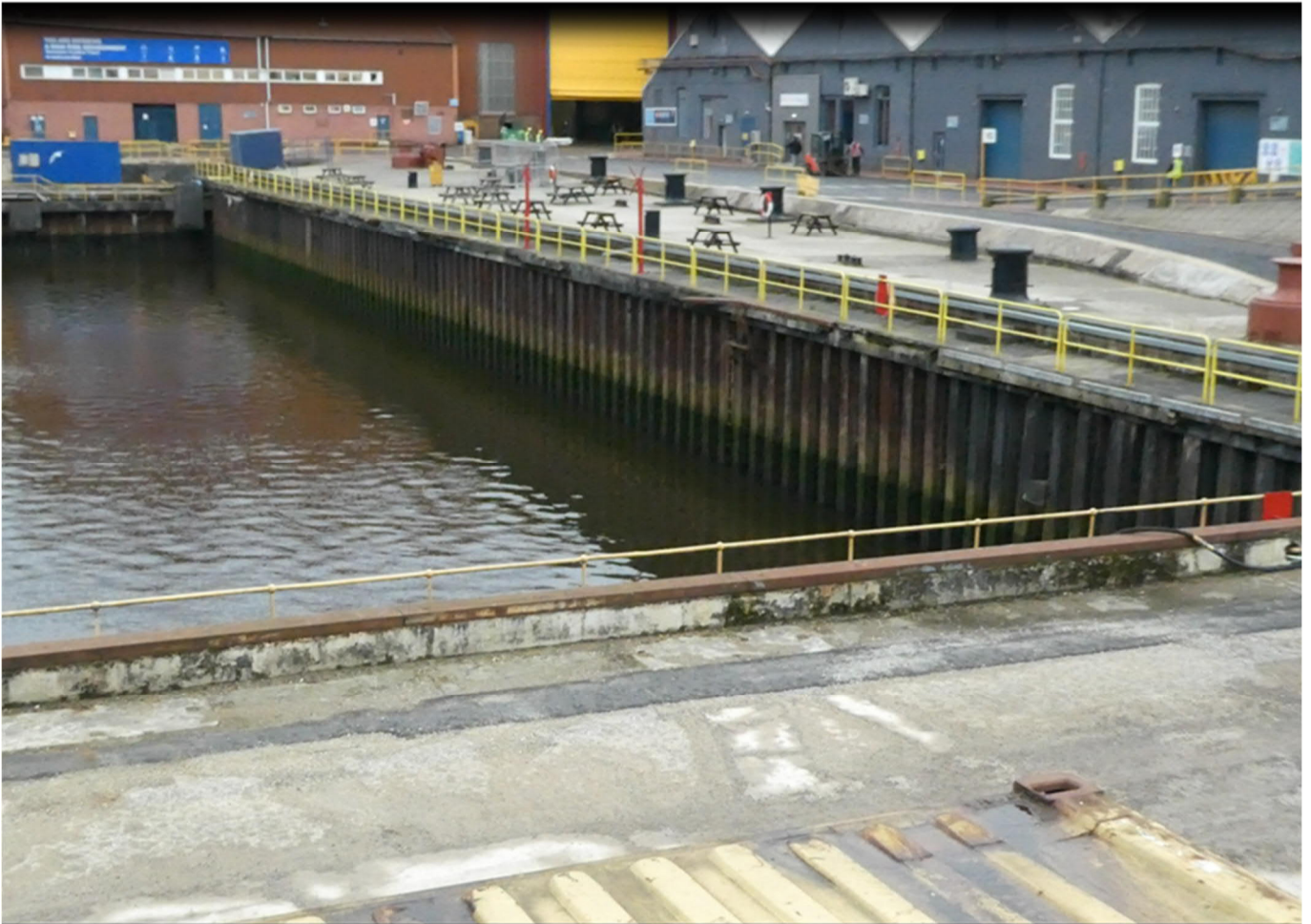
Photo B.2: View of Wet Basin and southern quay wall, taken from western quayside
