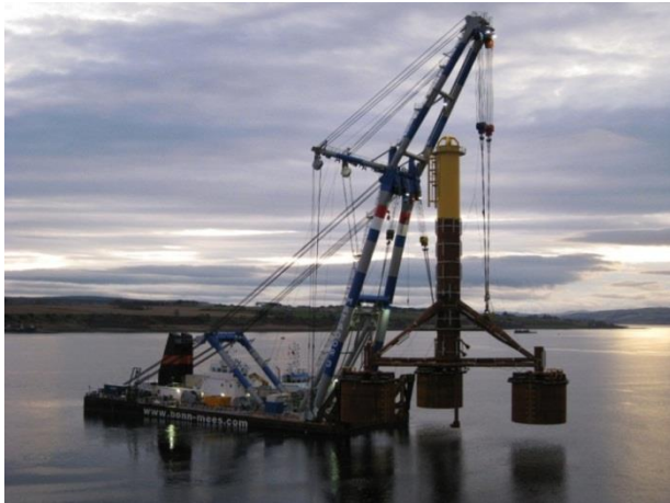
Figure 7.22: An Oil and Gas Platform with Suction Piles (Source: Ithaca)
