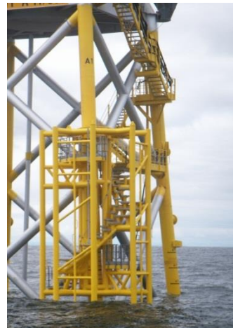
Figure 7.15B: Close Up View of the Representative WTG Access System
