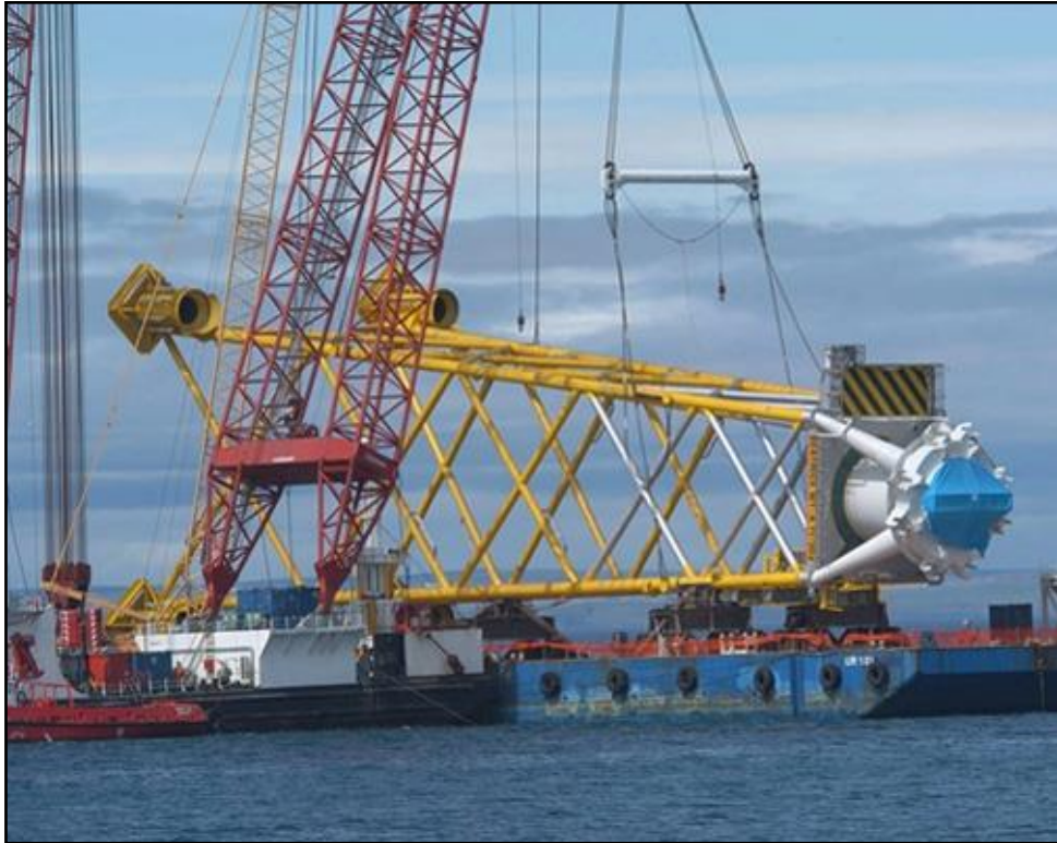
Figure 10A.6.6 The jacket structure used at the Beatrice OWF demonstrator site, Moray Firth.
