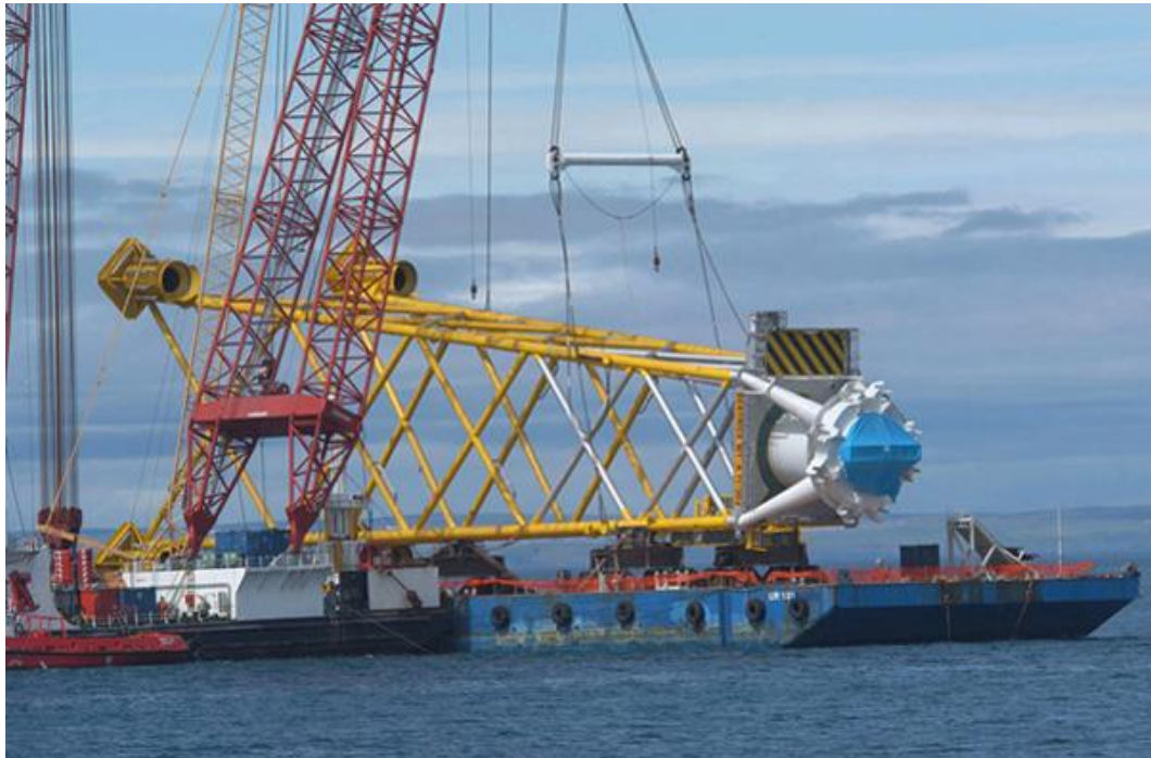
Figure 10A.5: Photo of the jacket foundation used at the Beatrice Demonstrator Project
