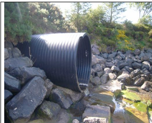
G2 Running freshwater exits from large culvert onto beach, to east of existing pier. Photo 81.
