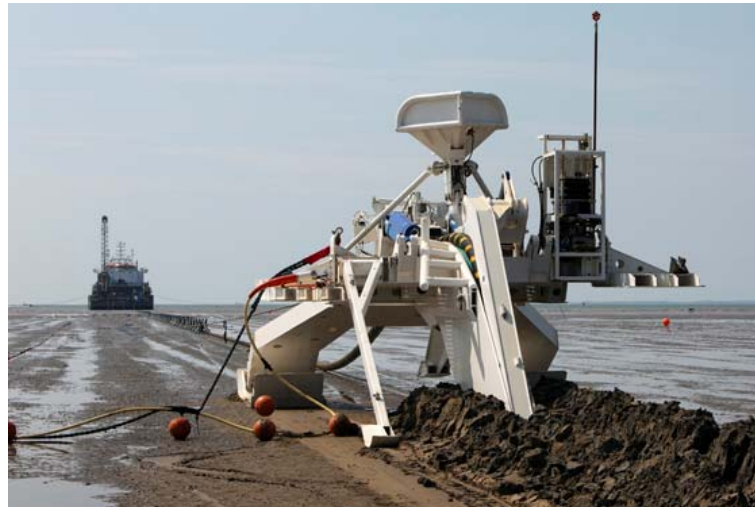
Figure 8.1 Typical Cable Plough
