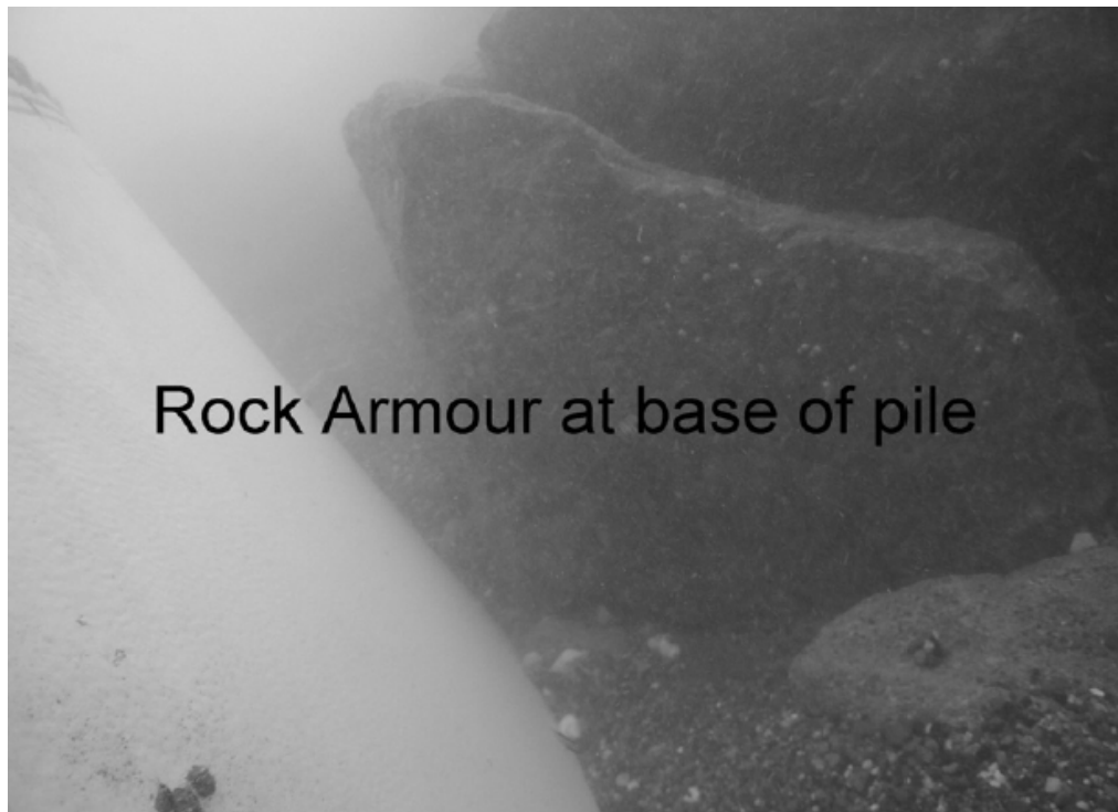
Figure G- 8 : Underwater photograph of rock armour at the base of a structure. Source: Whitehouse et al., (2011)
