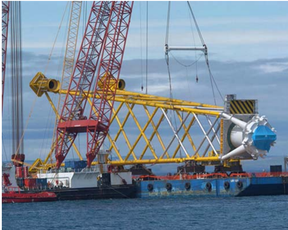
Figure G- 3: The jacket structure used at the Beatrice OWF demonstrator site, Moray Firth
