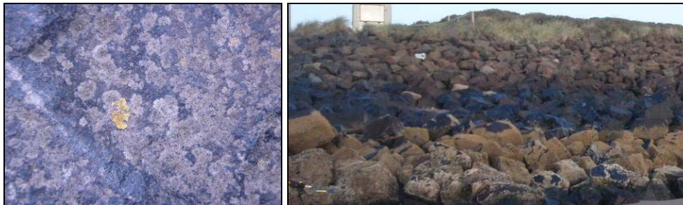
Plate 4.26 Lichen covered boulders of the rock revetment (left photo: grey and yellow lichens, right photo: black band of lichens)
