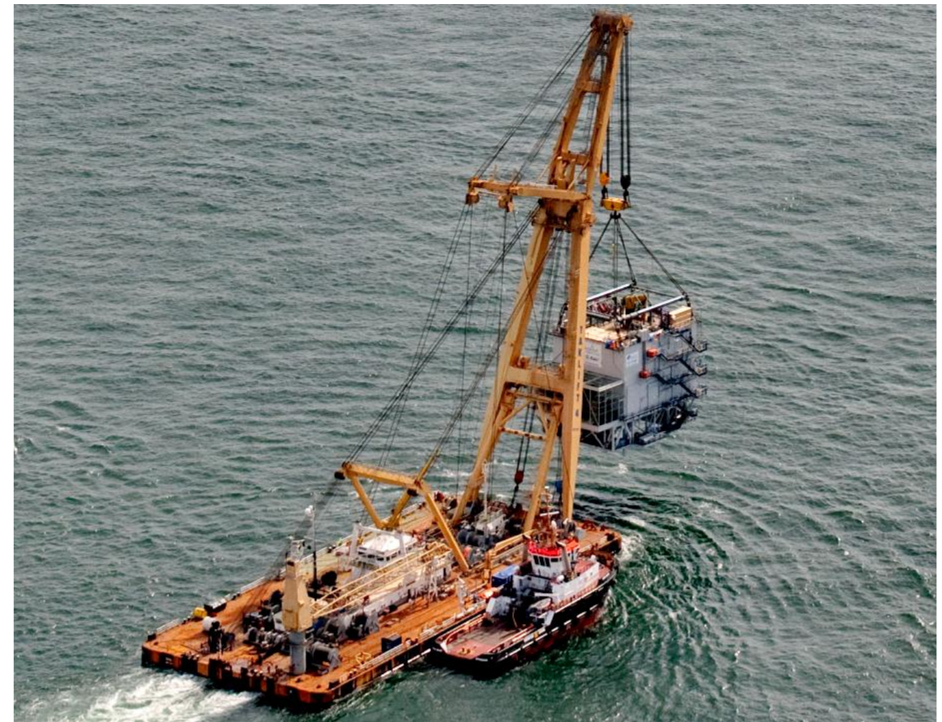
Figure 5.10: Sheerleg barge Taklift transporting substation topside (Picture courtesy of CG. Copyright ©vanoordbv-mennomulder.com)
