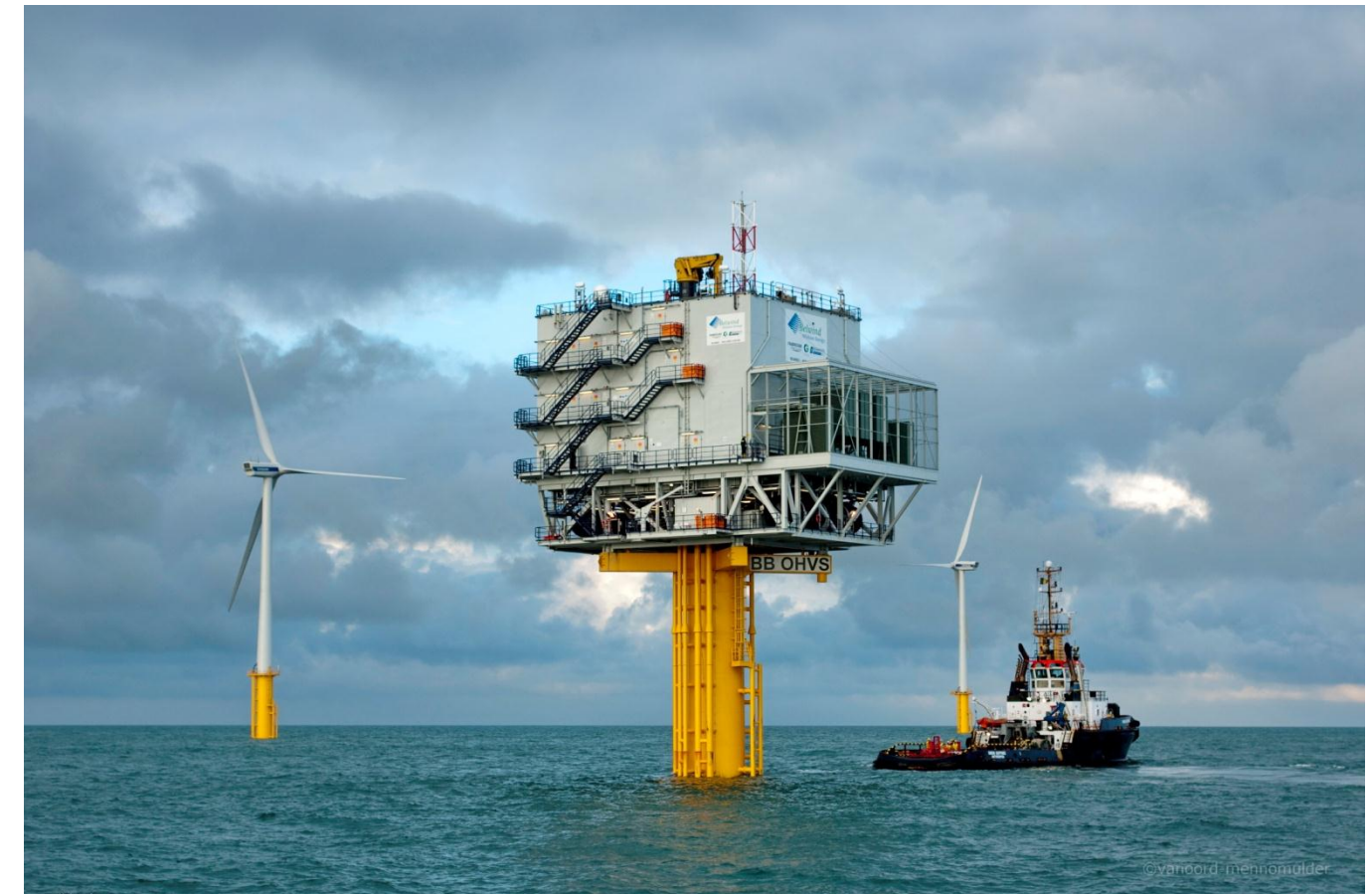
Figure 5.27: Installed substation (Pictures courtesy of CG. Copyright ©vanoordbv-mennomulder.com)
