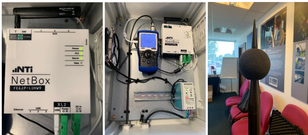
Figure 1 - Permanent Noise Monitoring Equipment
