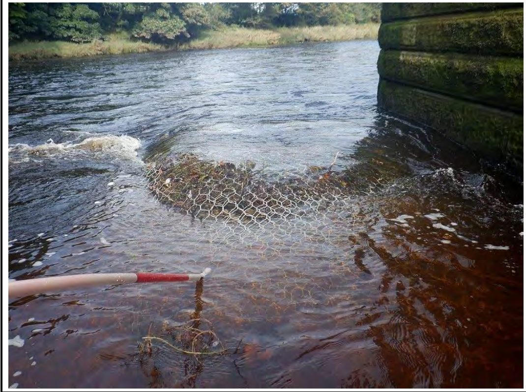
PHOTO 7: P7- PIER 3 DAMAGED GABIONS 14/09/20
