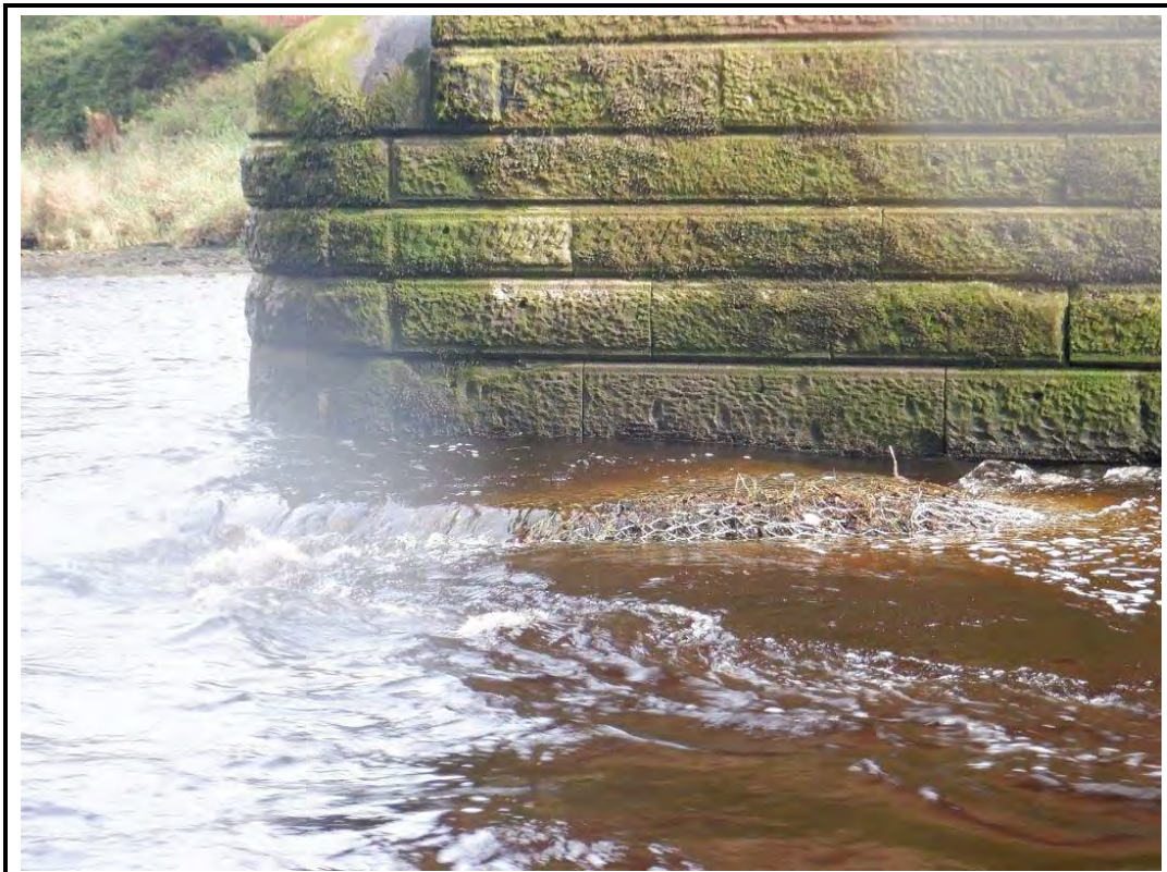
PHOTO 6: P6- PIER 3 DAMAGED GABIONS 14/09/20
