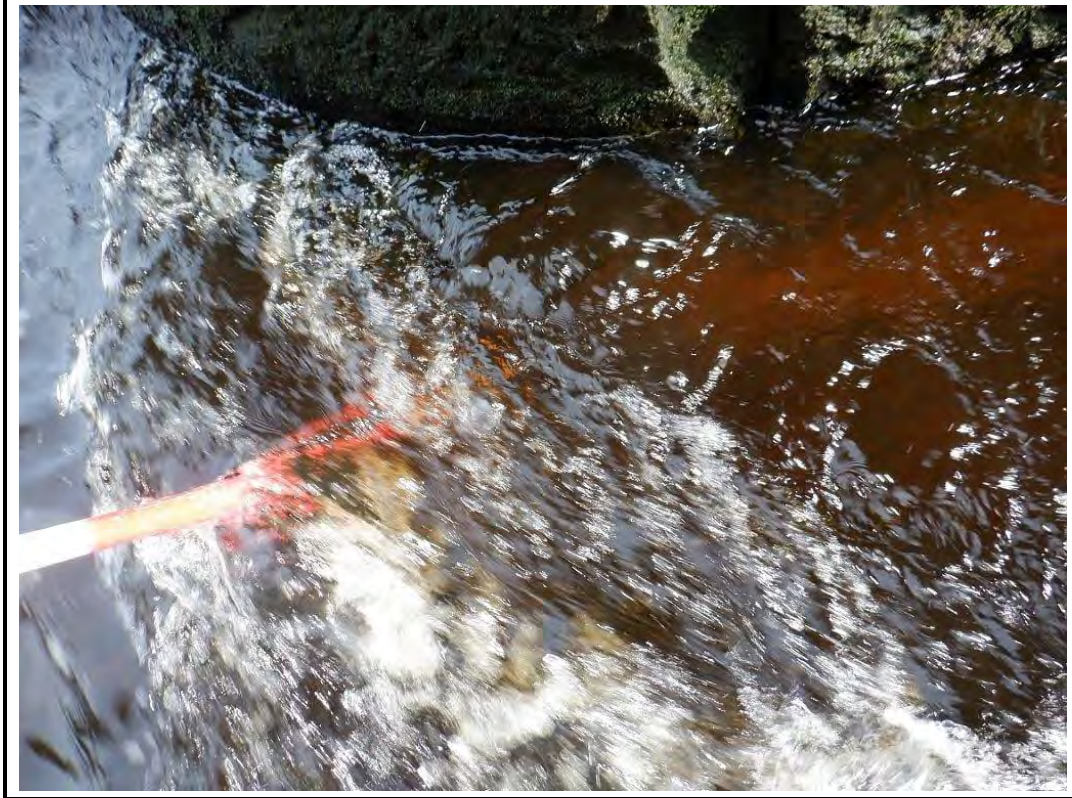
PHOTO 5: P5 - DAMAGED GABIONS 14/09/20
