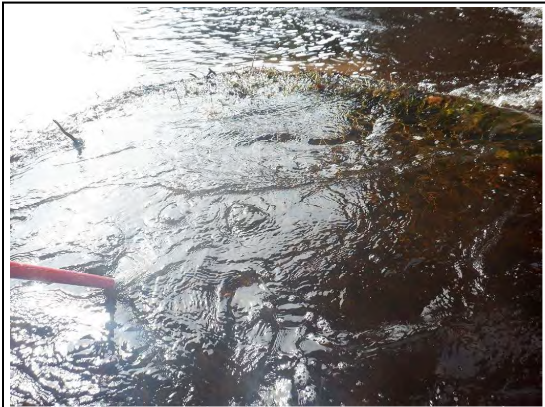
PHOTO 8: P8- PIER 3 DAMAGED GABIONS 14/09/20
