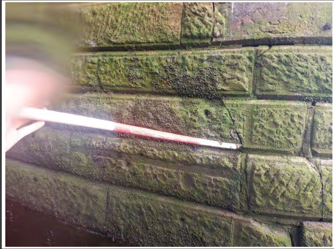
PHOTO 29: P29 - 2NO VERTICAL FRACTURES 14/09/20
