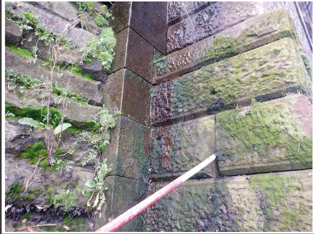
PHOTO 21: P21 - DOWNSTREAM RETURN - FRACTURE 14/09/20
