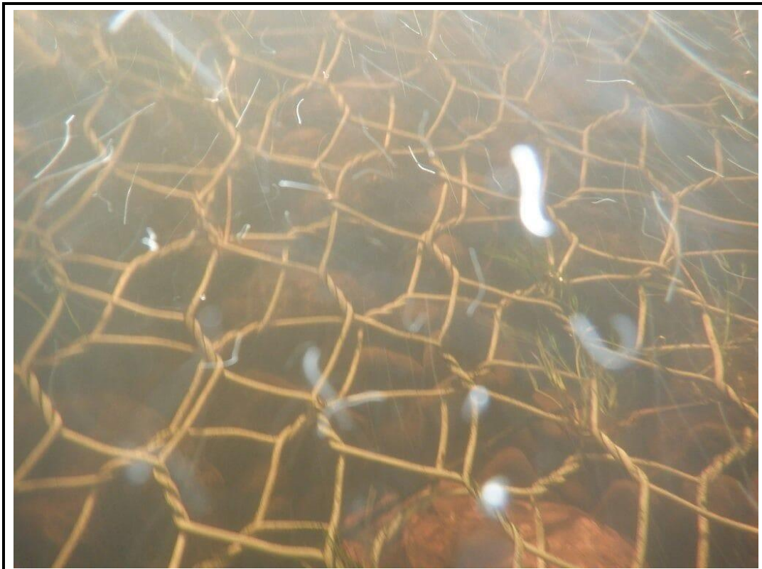
PHOTO 10: P10- PIER 3 DAMAGED GABIONS 14/09/20
