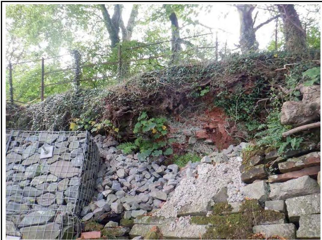
PHOTO 12: P12 - EROSION UPSTREAM LOW MILEAGE AFTER THE GABION BASKETS 14/09/20
