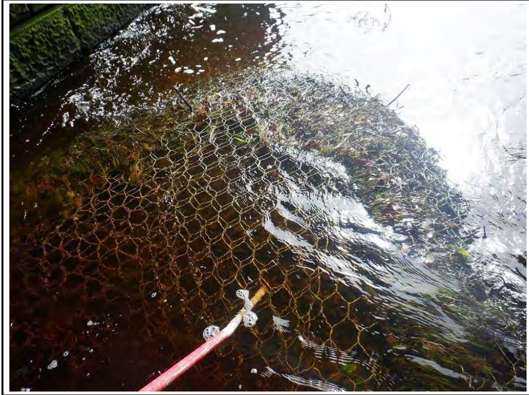
PHOTO 9: P9- PIER 3 DAMAGED GABIONS 14/09/20
