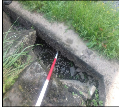
Key 3 - View of undercutting to the concrete apron upstream
