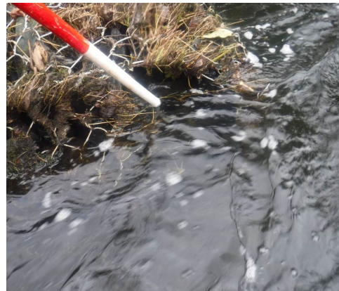
Key 5 - View of tear to the upstream LM gabion
