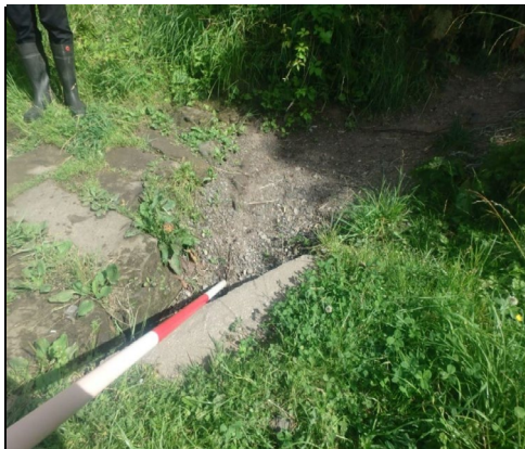
Key 4 - View of undercutting to the concrete apron downstream
