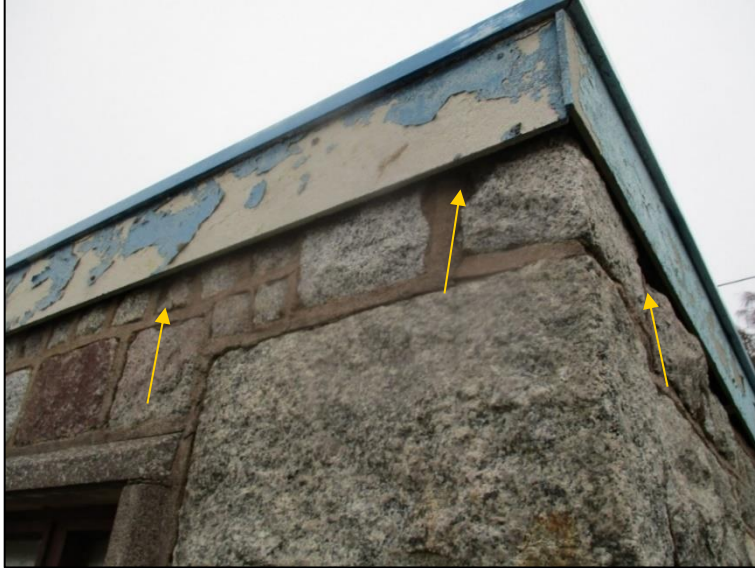
Photograph 6: Gaps between granite block work and roof fascia which may permit access by roosting bats.
