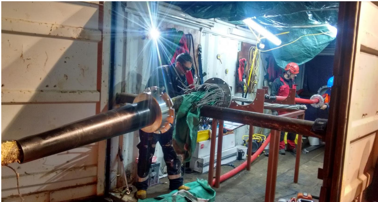
Figure 14. Orbital Marine Power and HV Contractors offshore on a multi-cat vessel cable jointing or “splicing” operations where static cables are permanently connected to the platform cable which supplies power and communications.
