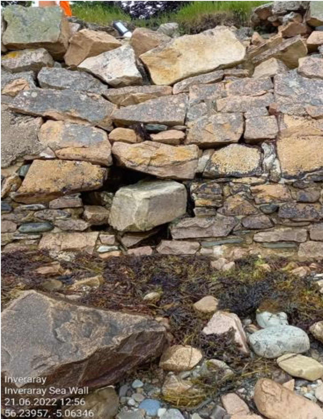
Ch.180 Wall collapse (No.2)
