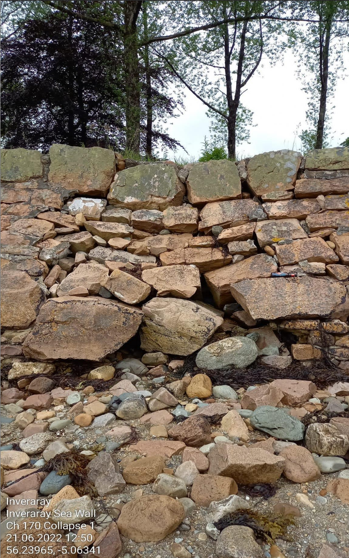
Ch.170 - Wall collapse (No.1)
