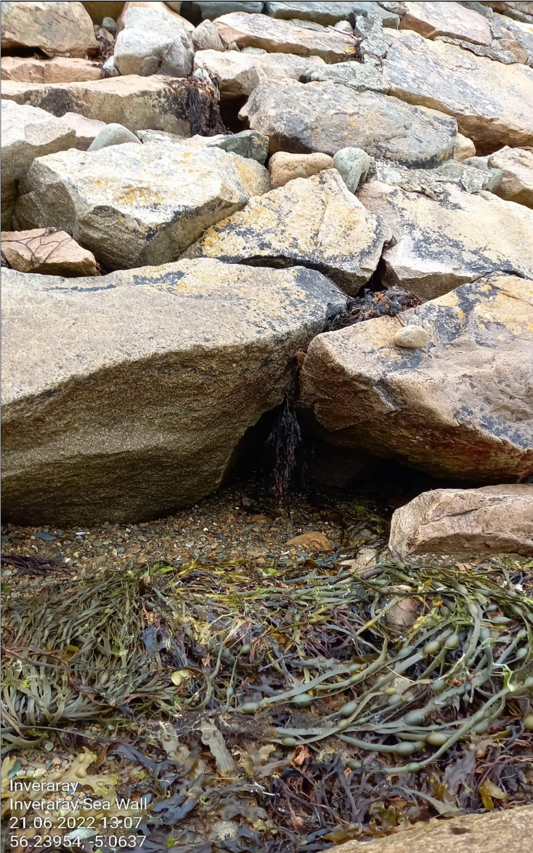
Ch.180 Wall collapse (No.3)
