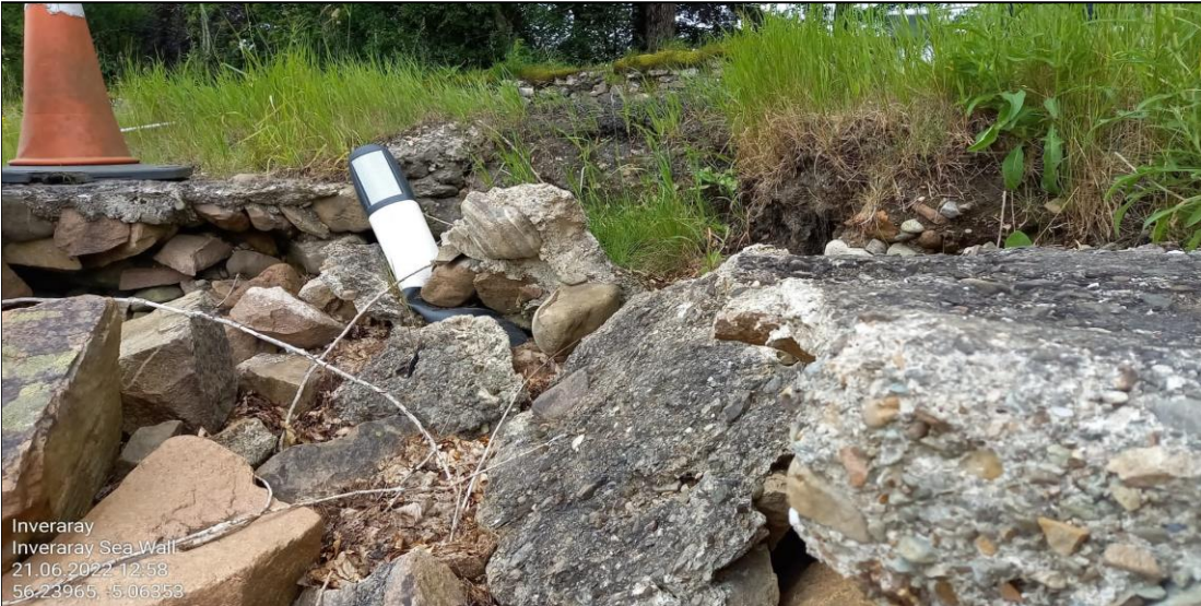
Ch.180 Wall collapse (No.3) - looking North
