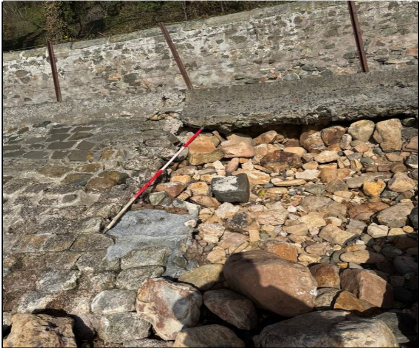
Key 2 -View of scour
