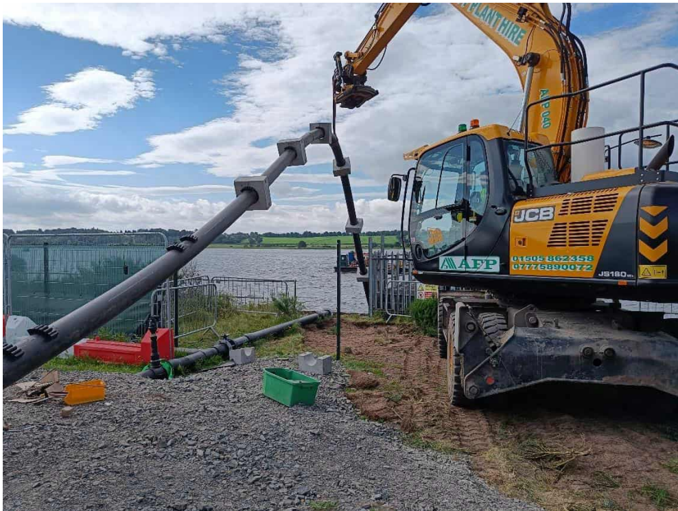
Figure 5 Offshore section lifted by Excavator JCB JS160 during positioning of the pipe on river bed
