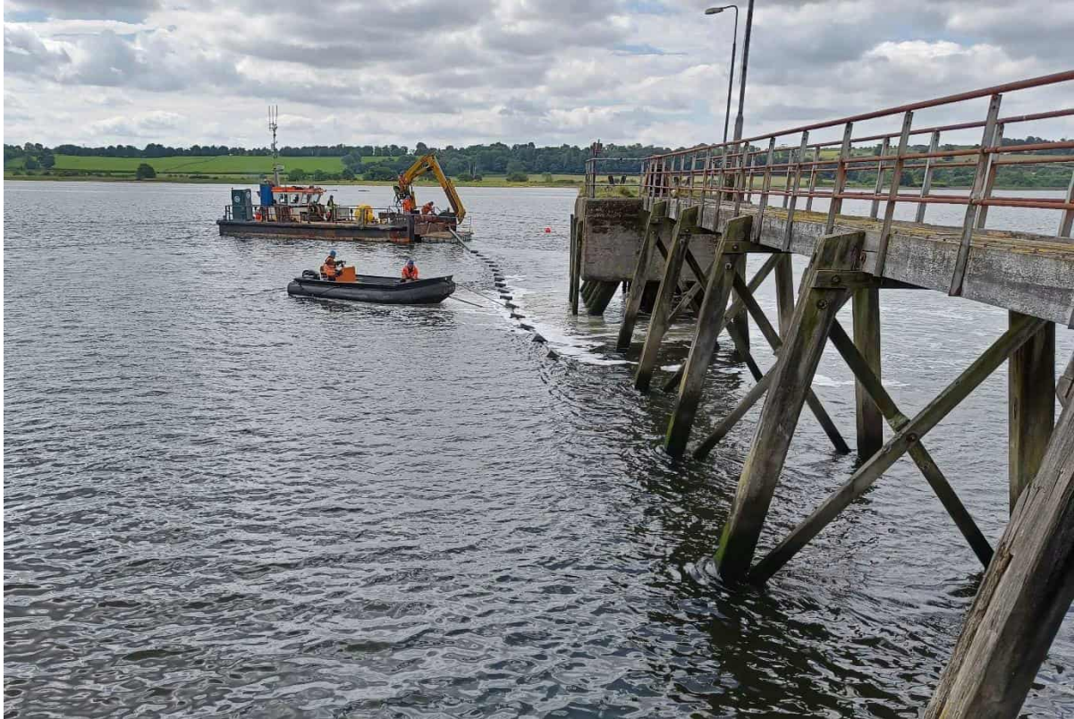
Figure 7 - Multi-Role Vessel “Mary M” and auxiliary boat used to install the discharge pipe at Bowling (June 2022)
