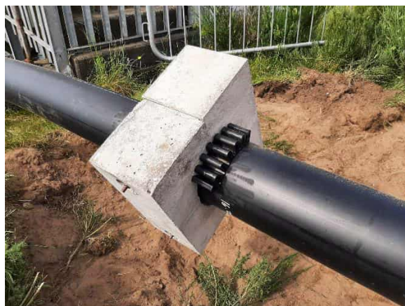
Figure 8 –Ballast concrete unit attached to the discharge pipe
