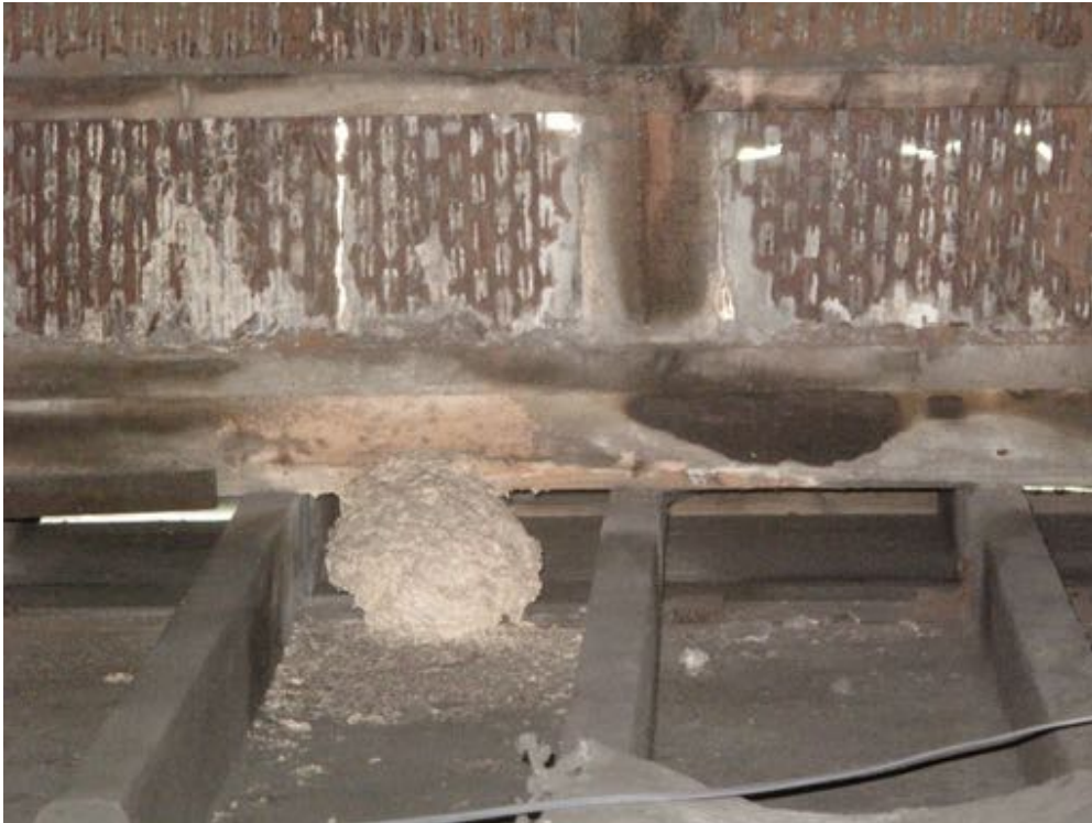
Photo 1 Wasp nest in northeast corner of attic. Light patches are holes in the roof.
