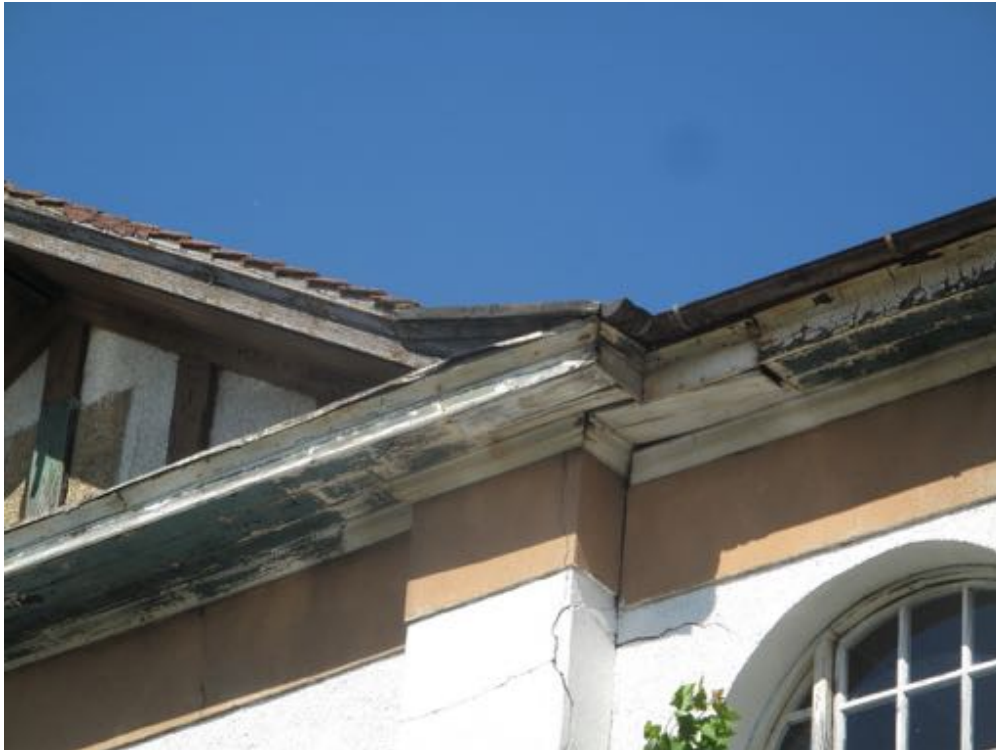
Photo 3. Gaps in the bargeboards, fascias & soffits
