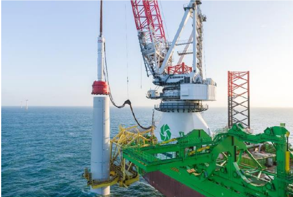
Figure 2-6: Example of the hammer being installed onto the top of the monopile.
