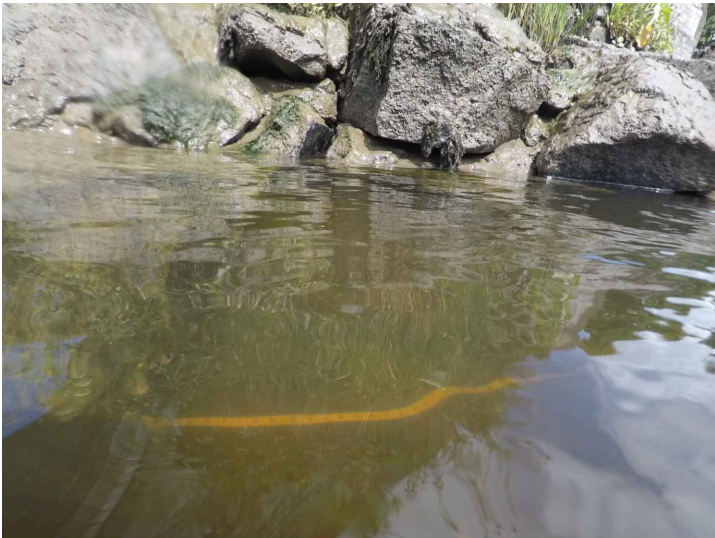
DEFECT 2: CENTRAL PIER – UNDERCUT TO THE OUTER FOOTING / SCOUR PROTECTION ON THE WEST SIDE OF THE PIER, 11.8m FROM THE TOE OF THE NORTHERN (UPSTREAM) SIDE
