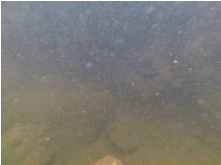
DEFECT 1: CENTRAL PIER – UNDERCUT TO THE OUTER FOOTING / SCOUR PROTECTION AT THE TOE OF THE PIER ON THE NORTHERN (UPSTREAM) SIDE
