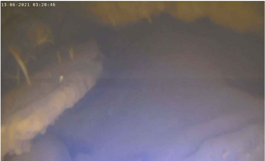
DEFECT 5: EAST PIER – UNDERCUT TO THE OUTER FOOTING / SCOUR PROTECTION, 11.0m FROM THE TOE OF THE NORTHERN (UPSTREAM) SIDE. THERE IS AN AREA 1200mm DEEP, 3m FROM THE START OF THE UNDERCUT
