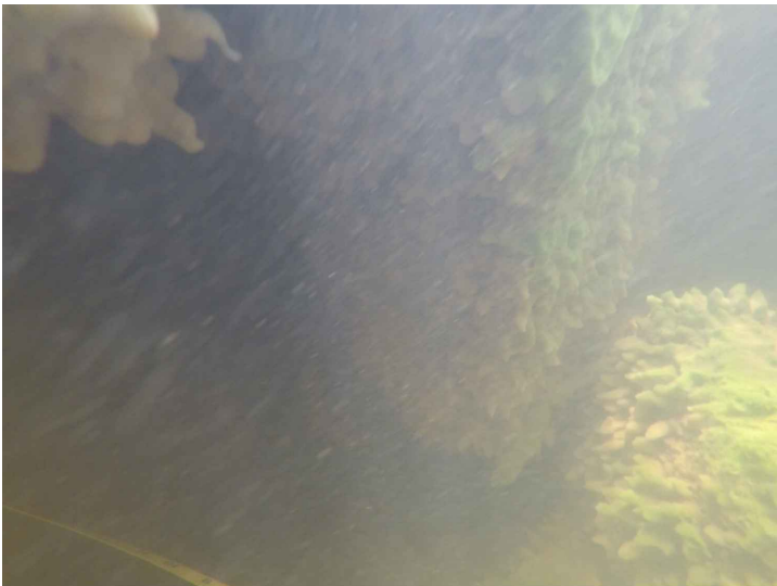
DEFECT 4: EAST PIER – UNDERCUT TO THE OUTER FOOTING / SCOUR PROTECTION AT THE TOE OF THE PIER ON THE NORTHERN (UPSTREAM) SIDE
