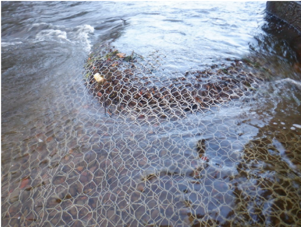
P07 - Deformed gabion baskets
