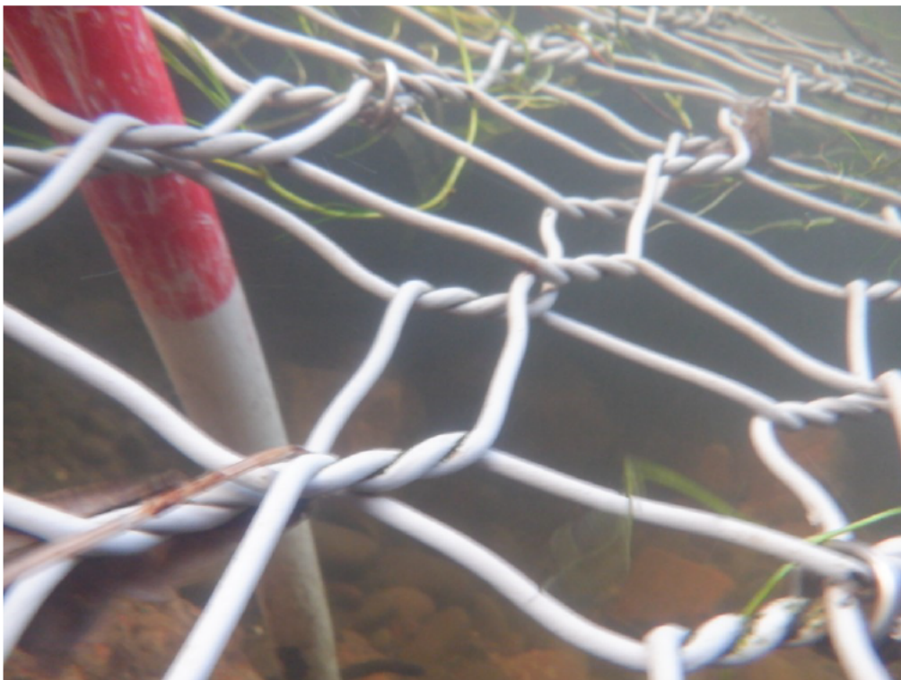
P08 - Loss of fill to gabions
