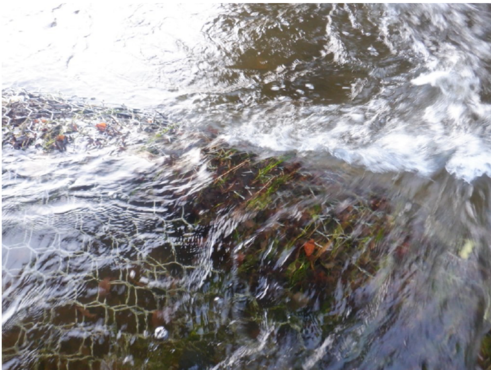
P06 - Deformed gabion baskets
