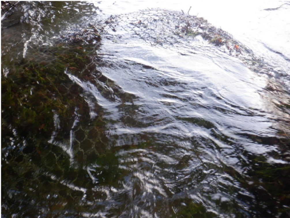
P05 - Deformed gabion baskets
