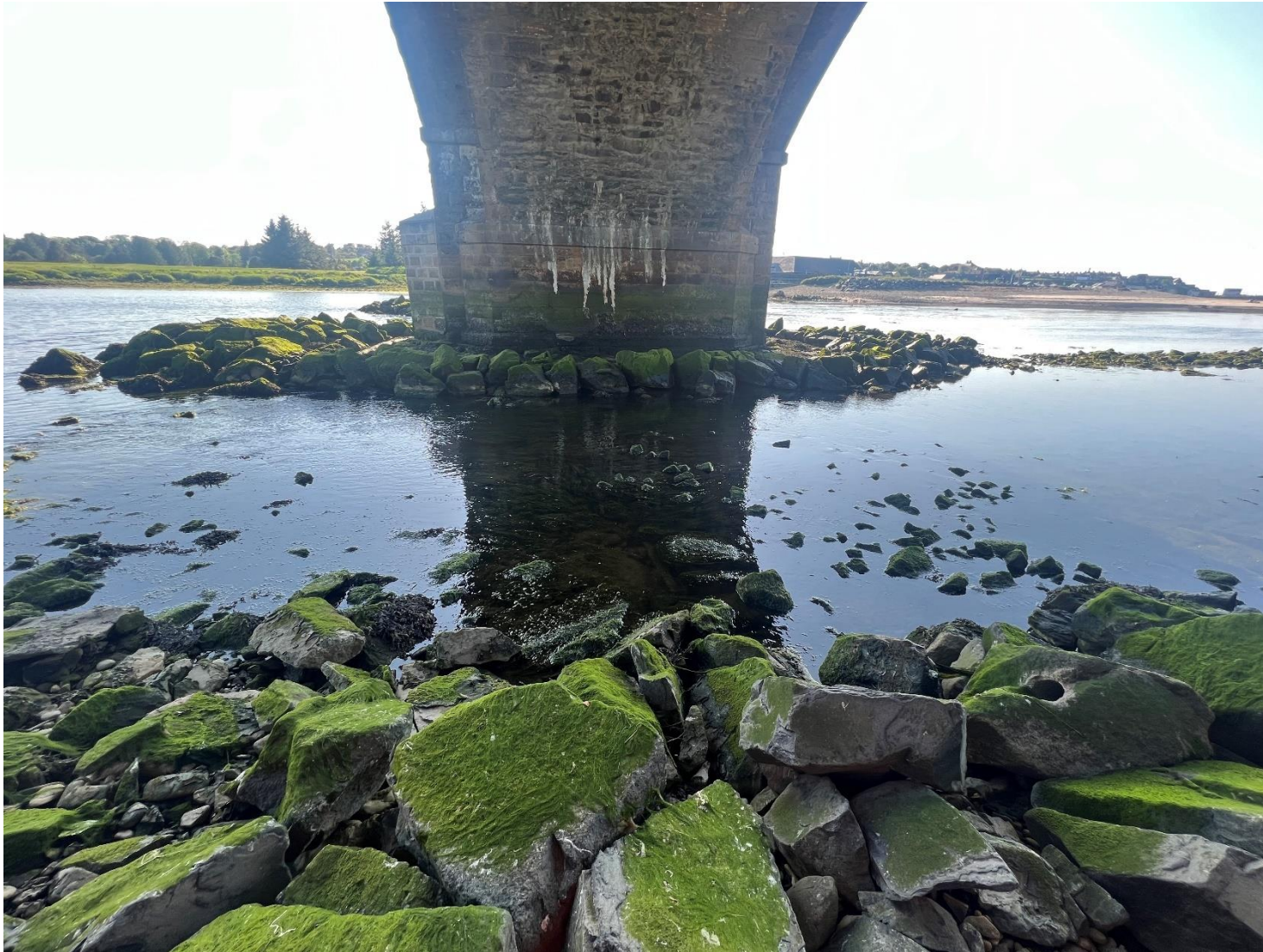
4.1.4 View looking west beneath a single span of Banff Bridge, showing existing rip-rap material surrounding the bridge
