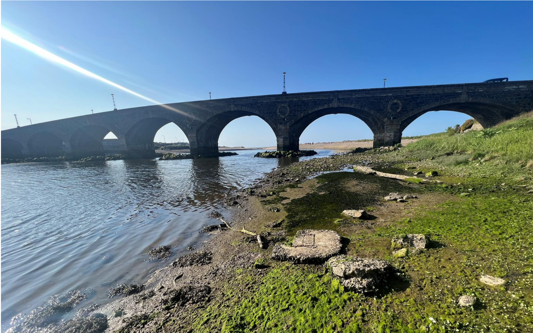
4.1.3 General View of Banff Bridge (taken from the southeast bank, looking north, and downstream)
