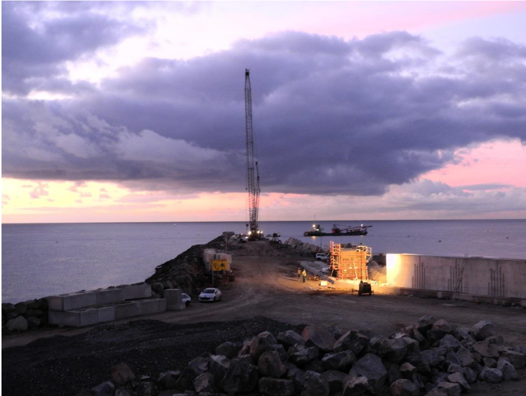
Figure 5.1: Example of Breakwater Construction Lighting
