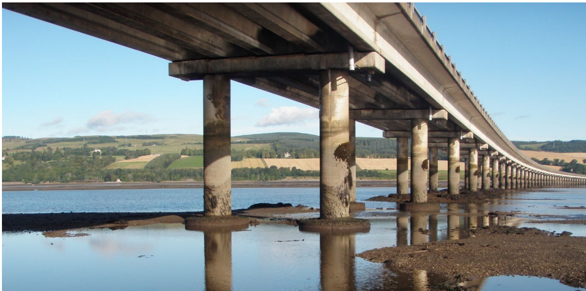
Figure 3, A9 Cromarty Bridge – Typical View below the Bridge - Piers, Crossheads and Bridge Beams.
