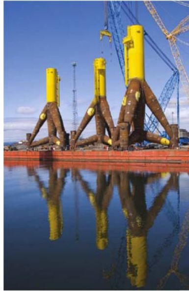
Figure 1 – Tripod support structures for Alpha Ventus under construction Source: Kaiser and Snyder (2012)
