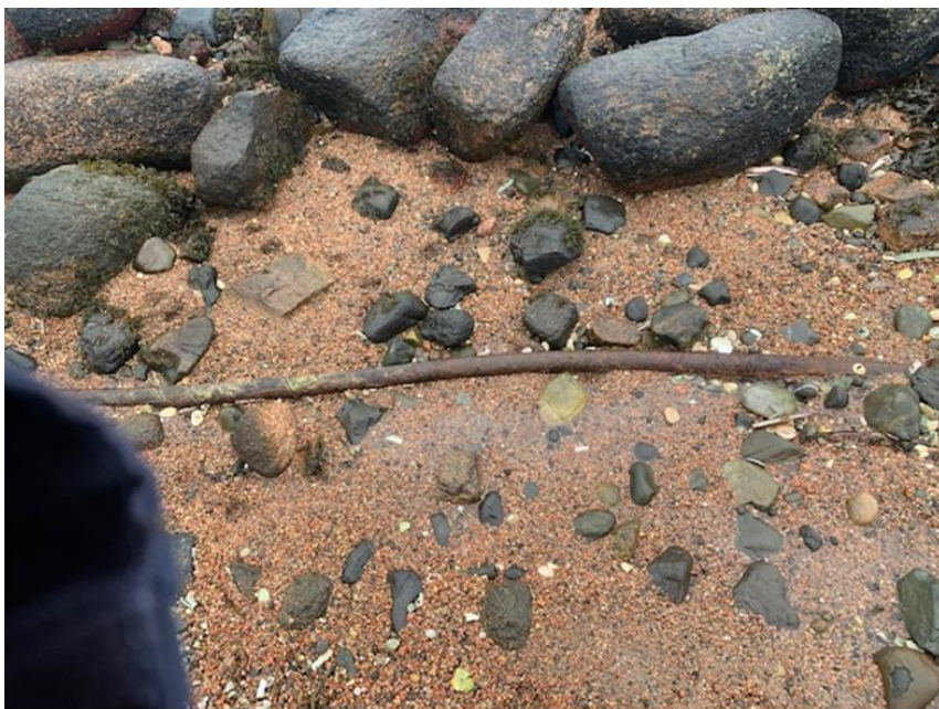
Figure 8 - Exposed cable at Mull landfall (Mull-Iona Island)
