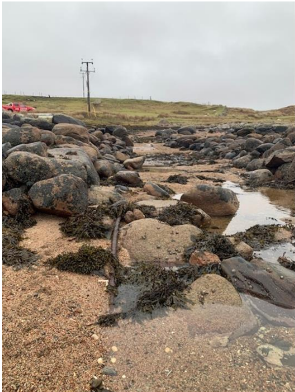
Figure 7 - Mull - Iona (Mull landfall) showing exposed cable
