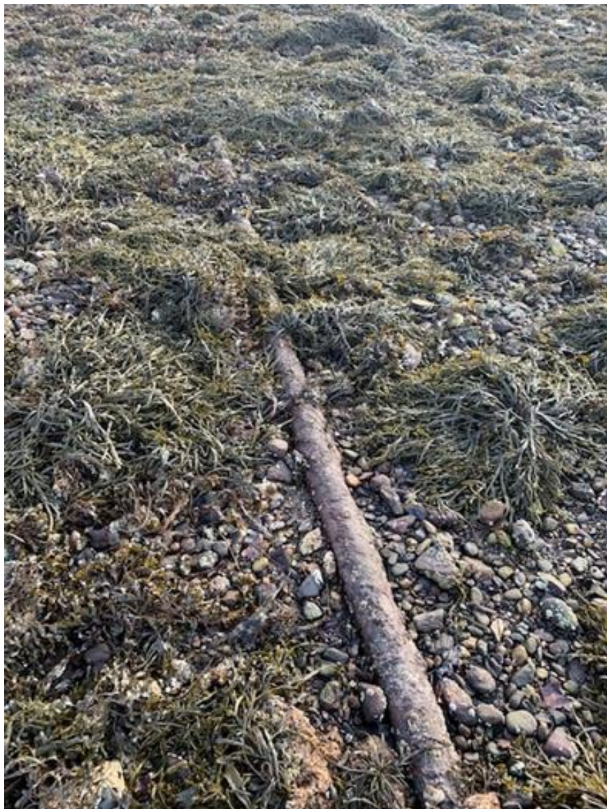
Figure 12 - Section of disconnected cable at Otter Ferry (N)
