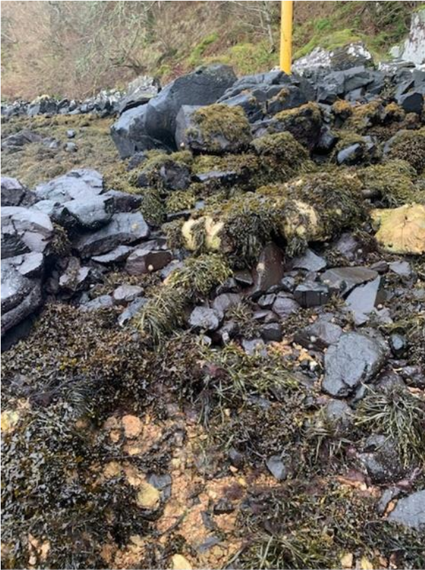
Figure 6- Exposed cable on Mull (Mull-Calve Island cable)
