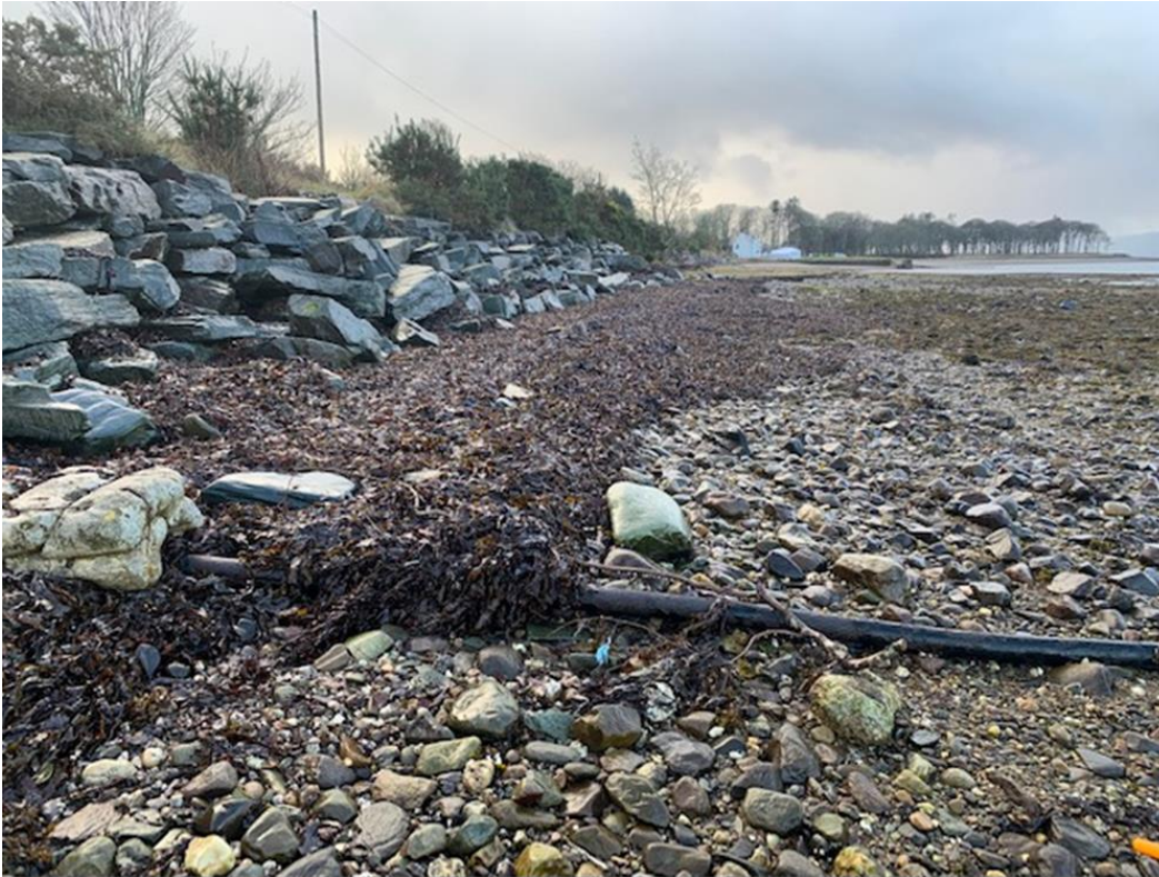
Figure 10 - Cable exposure at SSEN103 Otter Ferry
