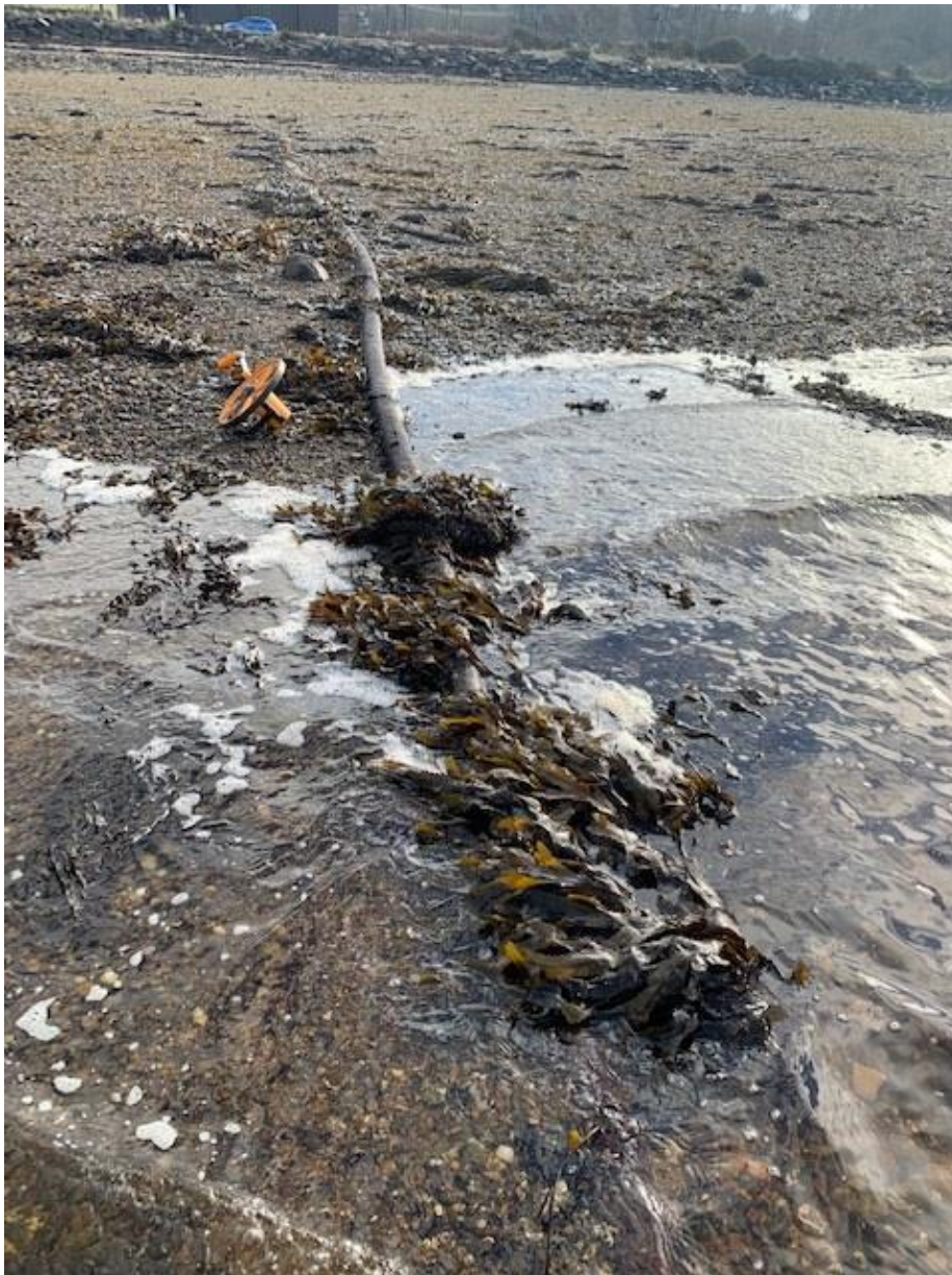
Figure 13 - Disconnected cable seen south of SSEN 103
