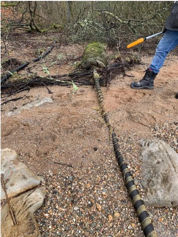
Figure 2 – Exposed cable above MLWS on Carrick Bay
