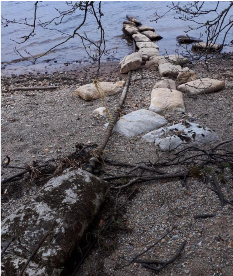
Figure 4- Exposed cable at low water Inchmurrin Island
