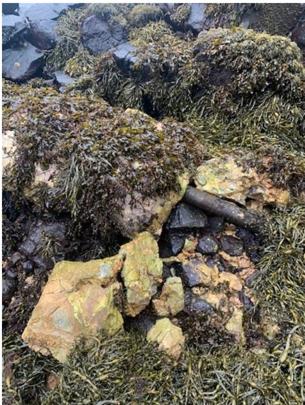
Figure 5- Remedial work required at Mull (Mull-Calve Island cable) broken concrete bags
