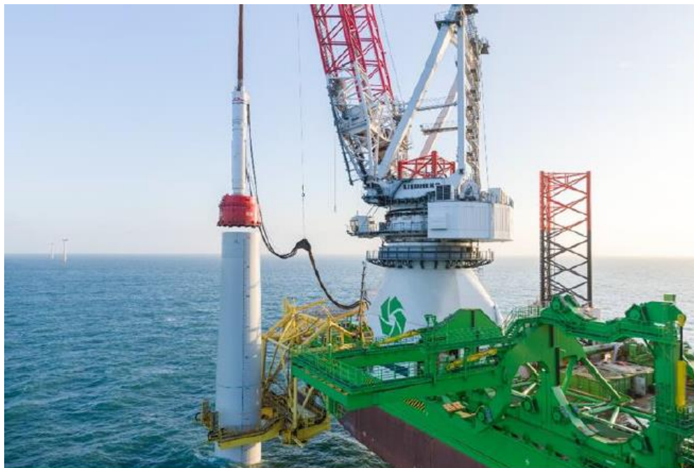
Figure 4-8: Example of the hammer being installed onto the top of the monopile.
