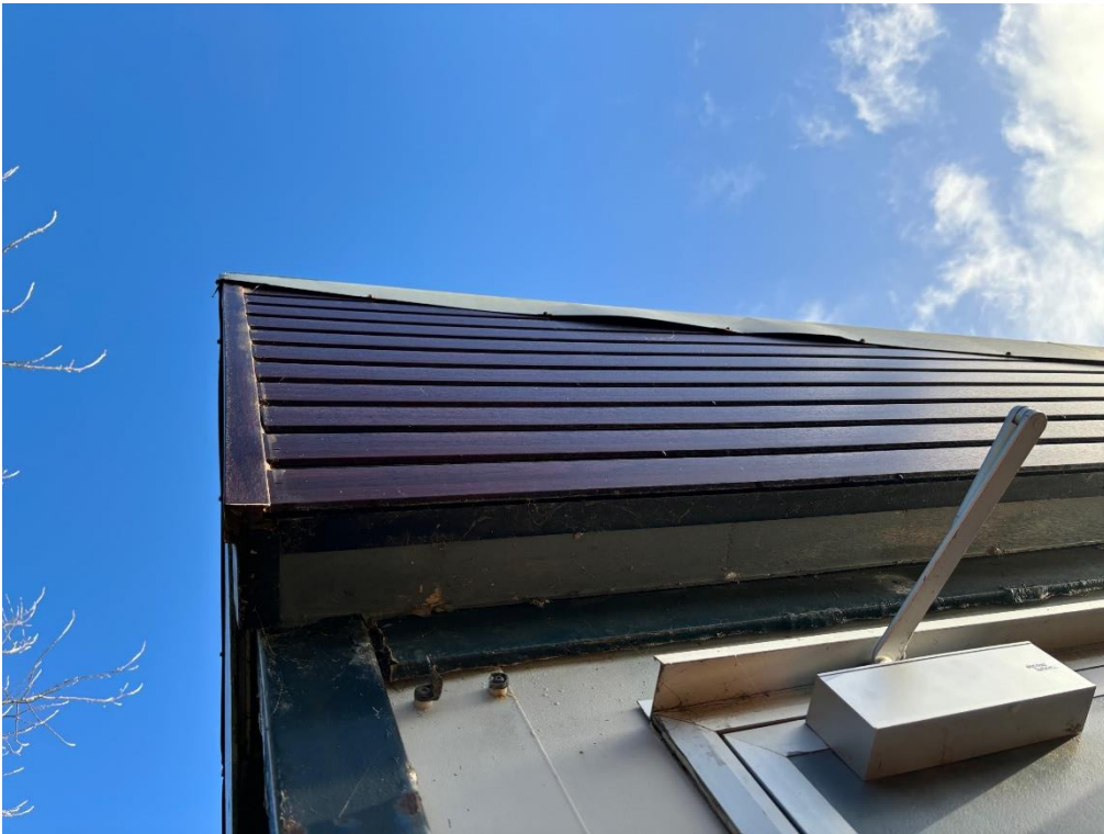
Photograph 15: PRF on toilet block
