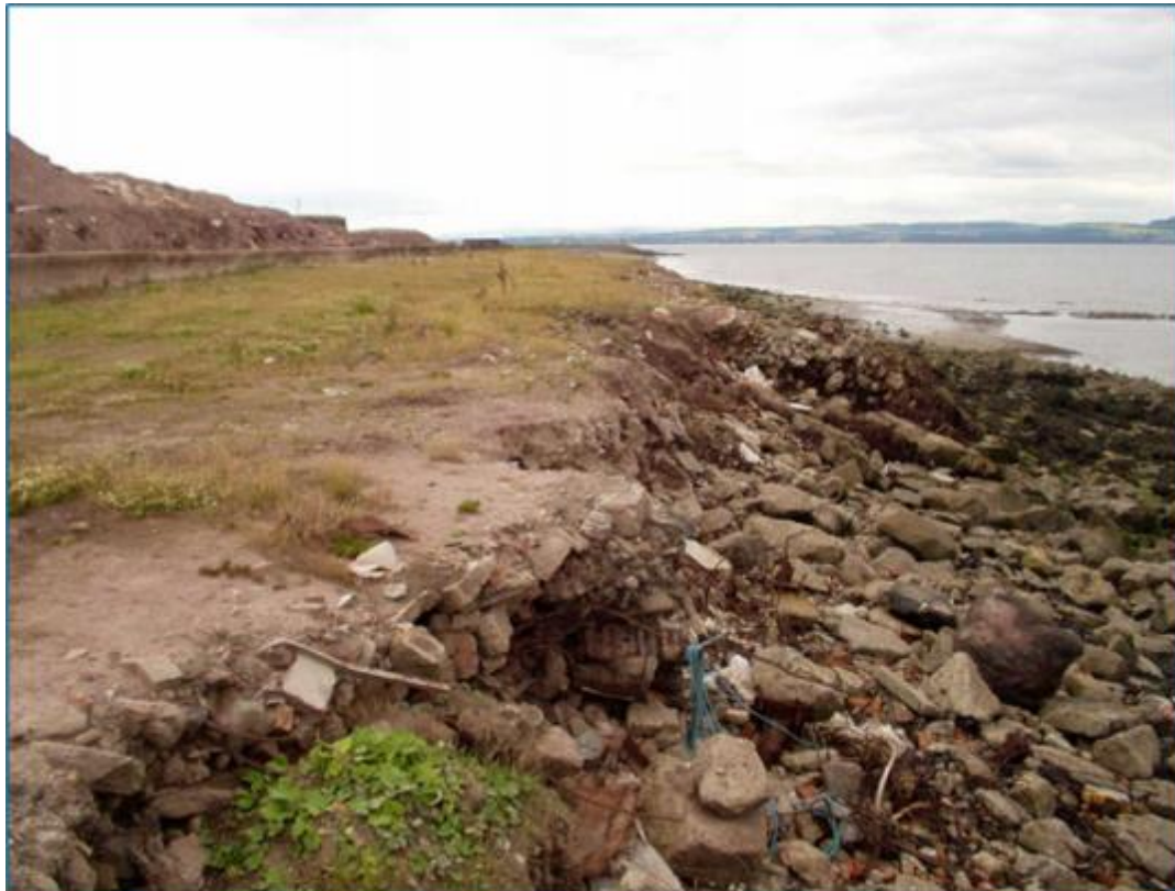
Figure 7-16 Eroding tipped building waste along Leith Sands (HR Wallingford, 2004)
