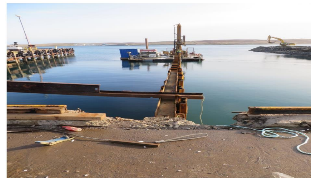
Plate 2-3: Photograph showing a tracked drilling rig set up for pre-treatment of bedrock
