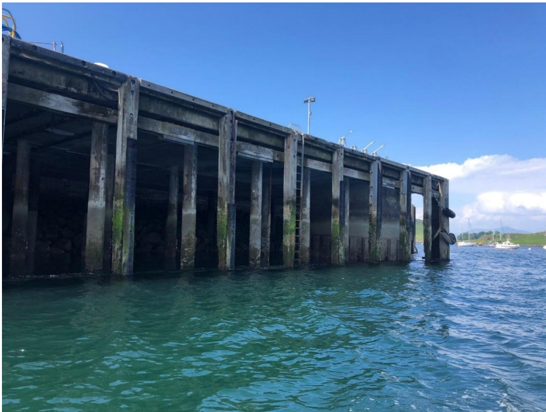
Photo 2: Close-up photo showing timber piles to be replaced like for like.
