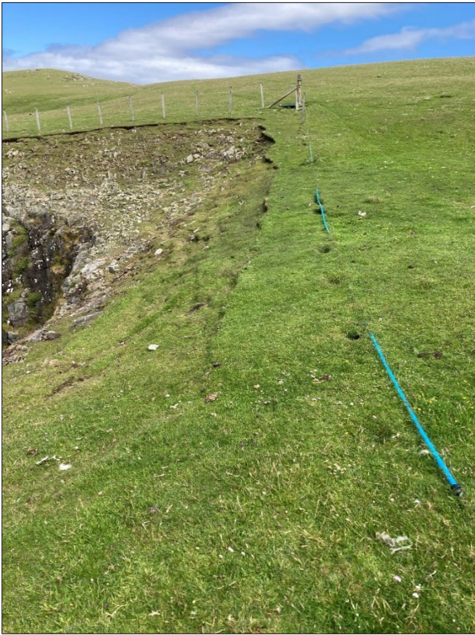
Plate 06: View of soil depths at the edge of the noust, facing north.
