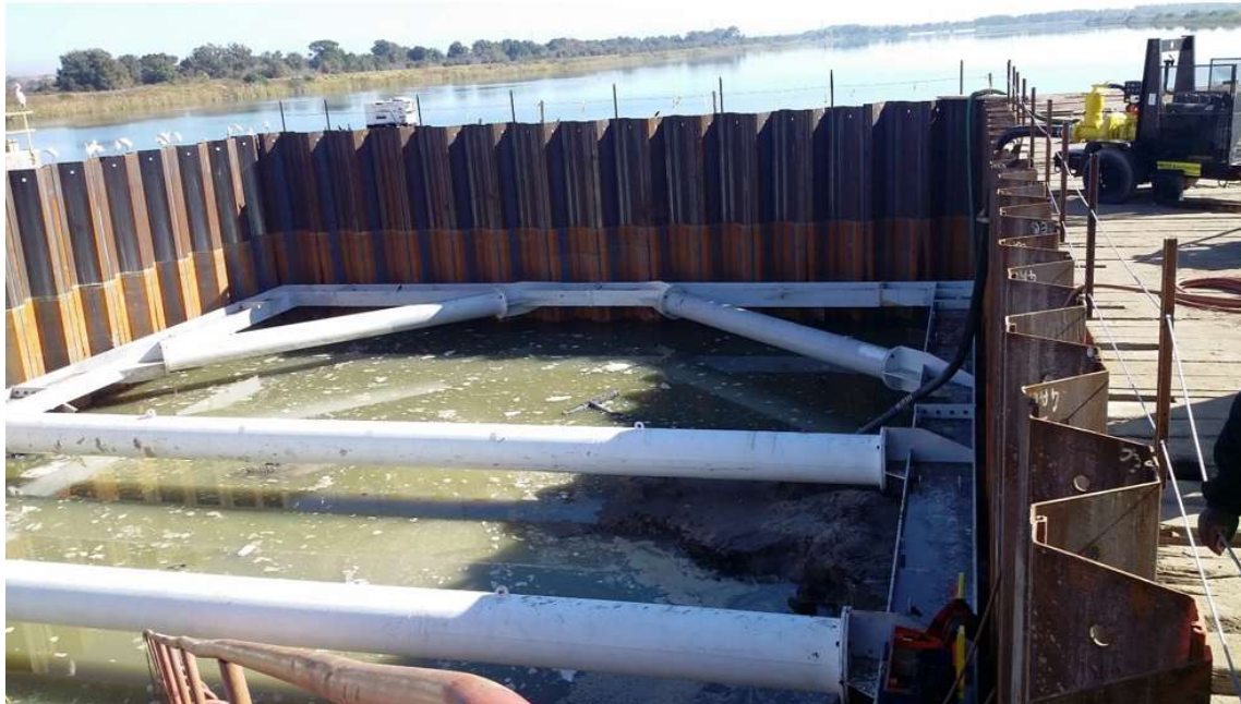
Figure 2.1: Example Image Showing Waling Beam, Props and Tie Rods within a Cofferdam
