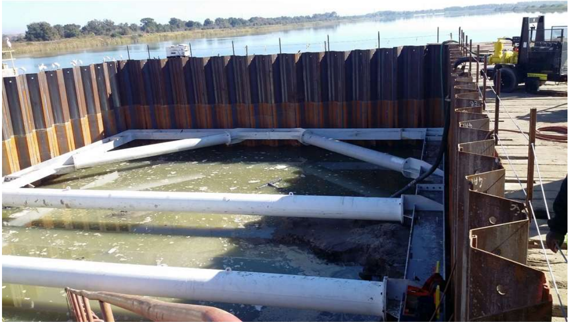
Figure 3.1: Example Image Showing Waling Beam, props and tie rods within a Cofferdam
