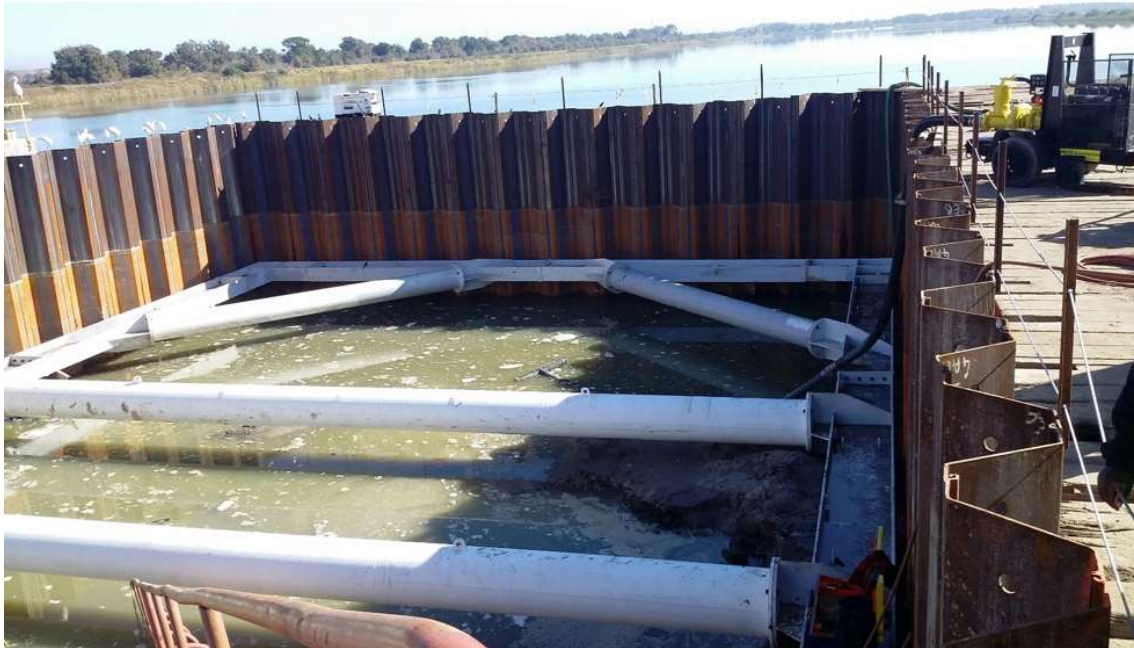
Figure 2.2: Example Image Showing Waling Beam, props and tie rods within a Cofferdam
