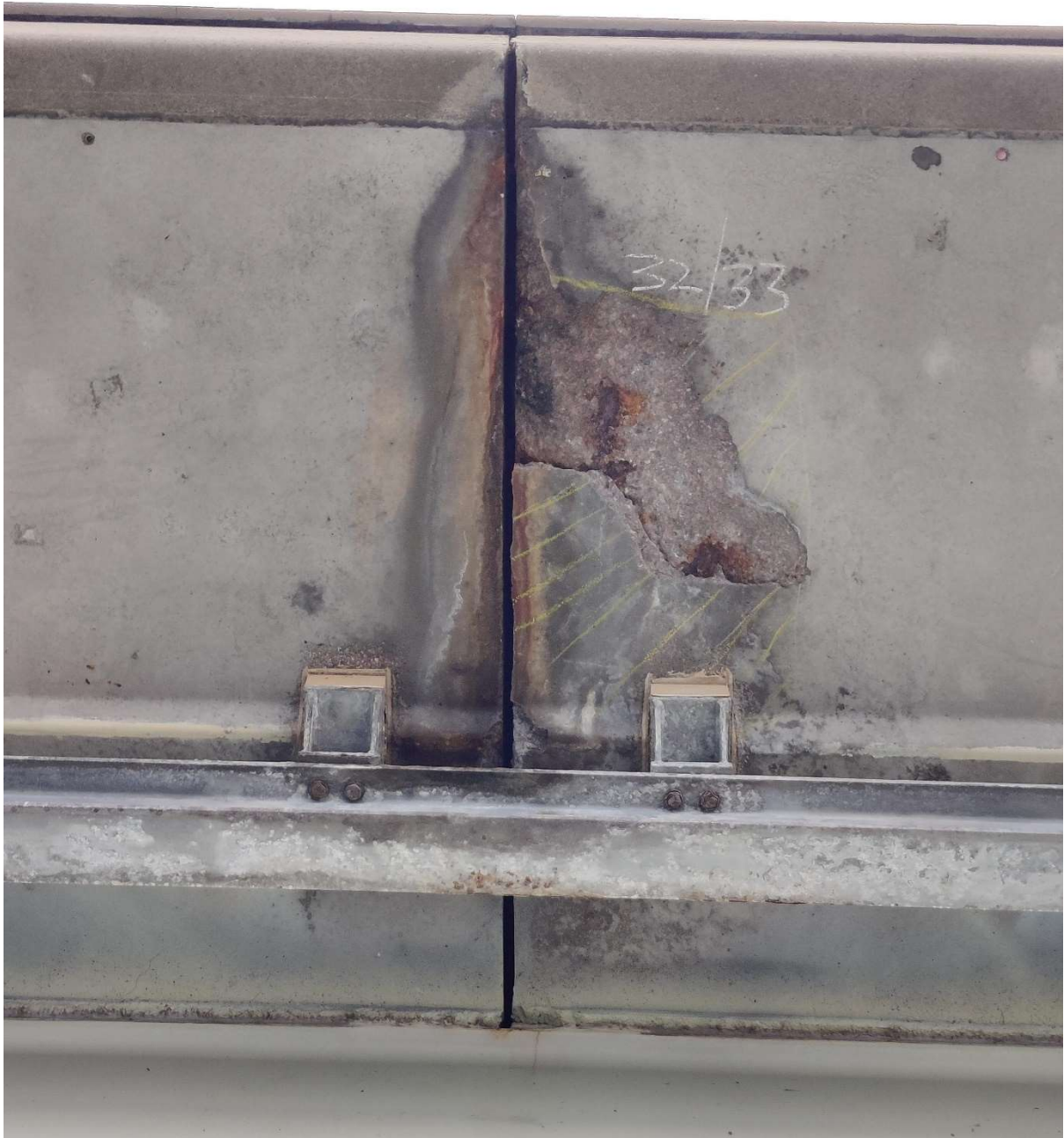
Typical defect to underside of concrete deck outer cantilever where proposed concrete repairs are proposed.
