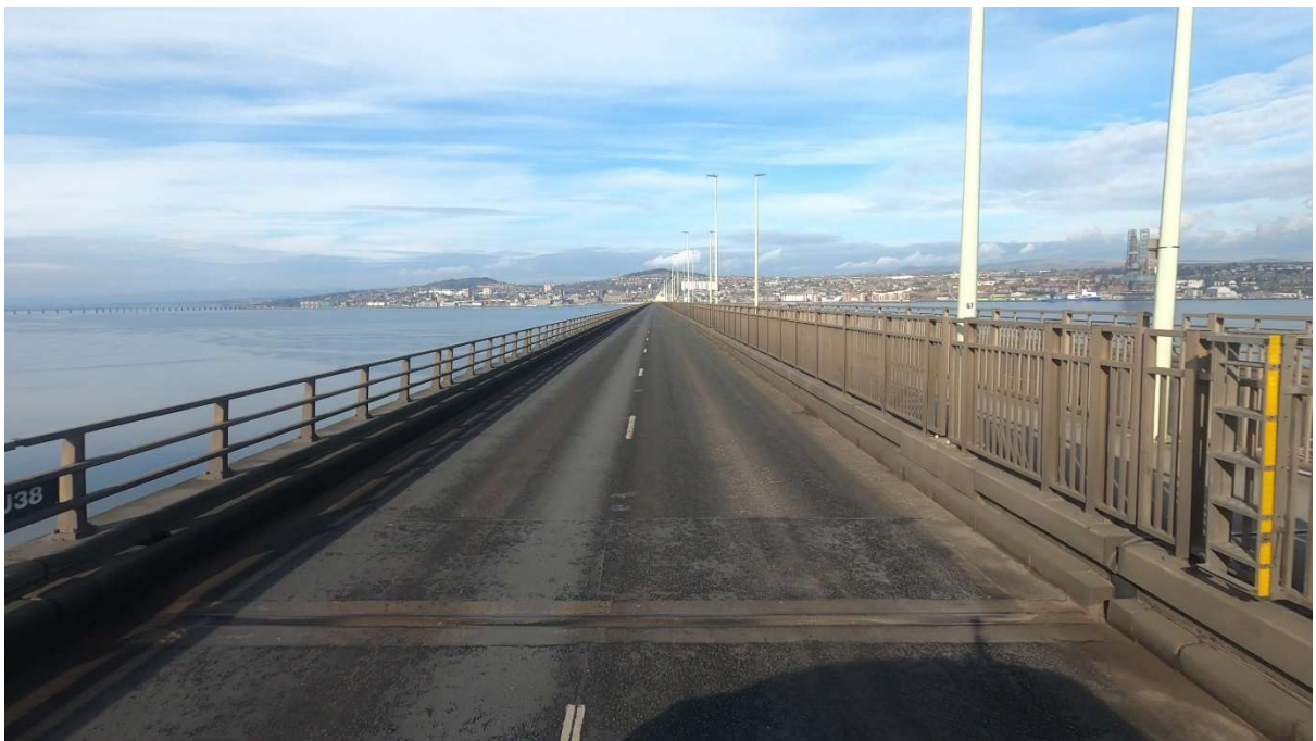
General View travelling Northbound showing existing worn surfacing and ageing expansion joint (looking Northwest)
