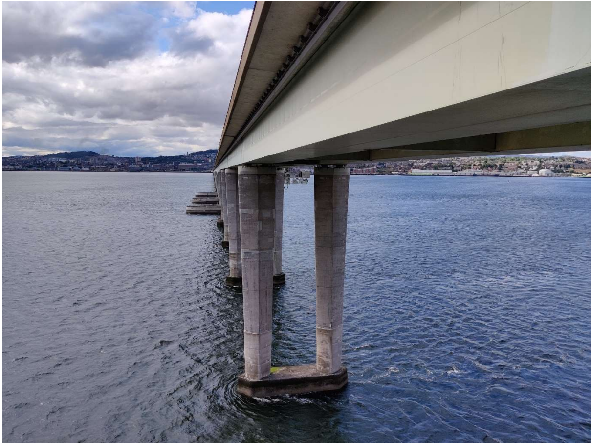
Typical View of Tay Road Bridge showing superstructure supported on reinforced concrete piers. Note outer concrete deck cantilevers where concrete repairs are proposed. See below for typical defect requiring repair.
