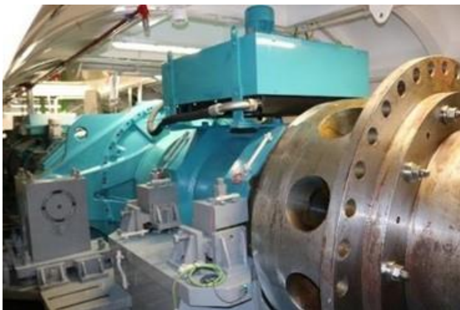
Figure 9: Gearbox in the Nacelle (Lower Block)
