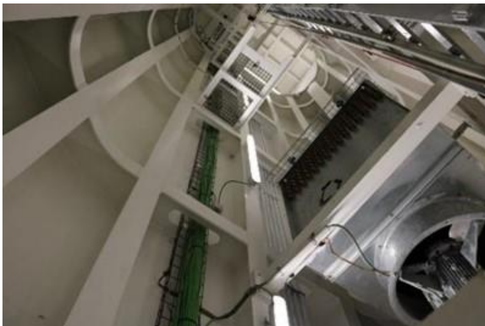
Figure 8: View Looking up into the Mast (Vertical Block) from the Nacelle (Lower Block)
