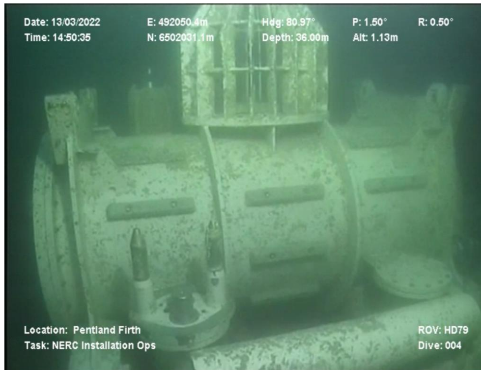
Figure 7 – Subsea hub showing guide pins and wet-mate plug
