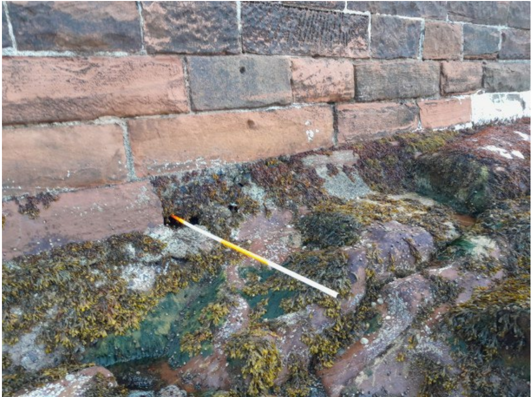
Photograph 23 - Section 3 - 9M 1416Y - Small void in concrete repair at toe 500mm deep- 18.06.23
