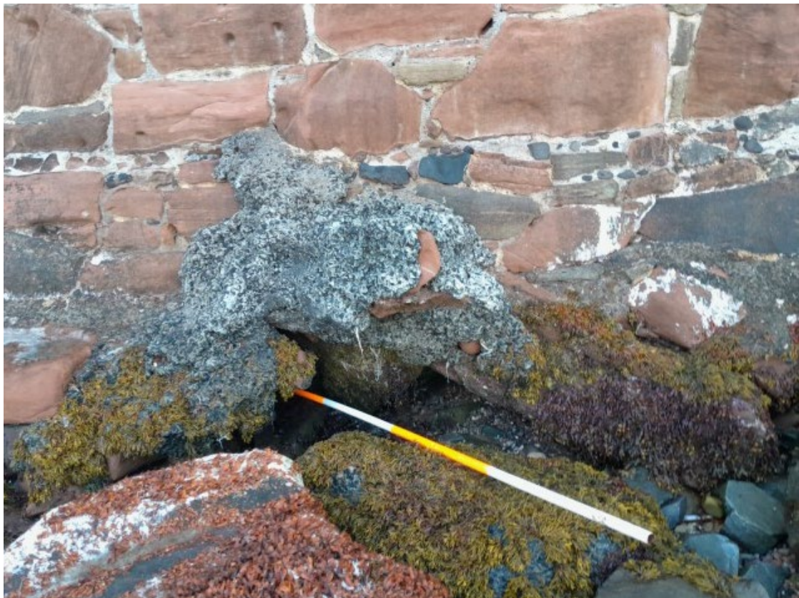
Photograph 17 - Section 3 - 9M 1395Y - Voids at toe of concrete repair no change (750mm) - 18.06.23
