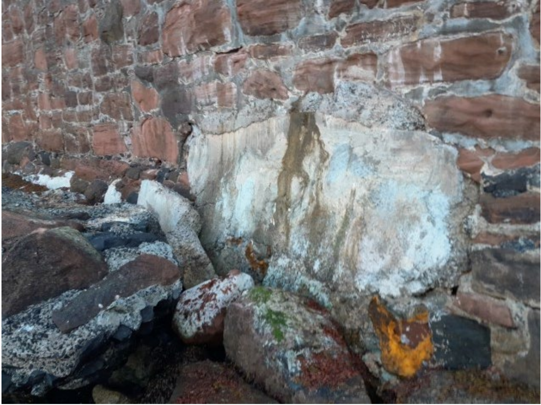
Photograph 18- Section 3M- 9M 1400Y- repair condition, void at toe of wall- 18.06.23
