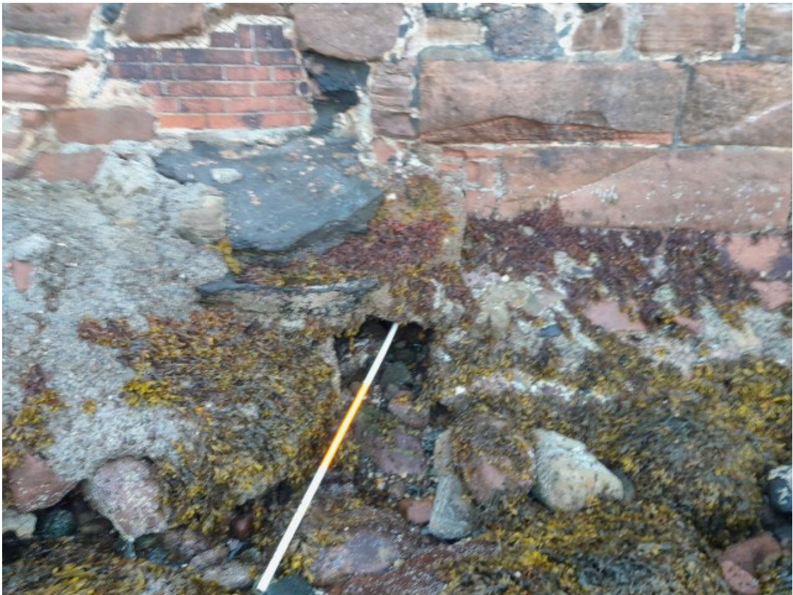
Photograph 22 - Section 3 - 9M 1414Y -void @ repair 750 deep- 18.06.23
