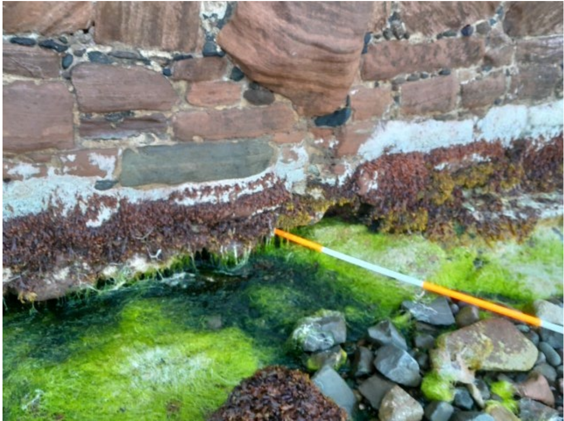
Photograph 16 - Section 3 - 9M 1359Y - Undermining at toe, majority of void filled shingle - 18.06.23
