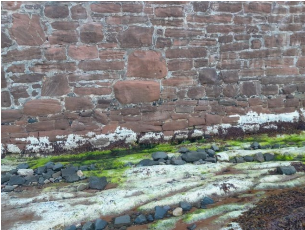
Photograph 14 - Section 3 - 9M 1328Y - Undermining at toe - 18.06.23
