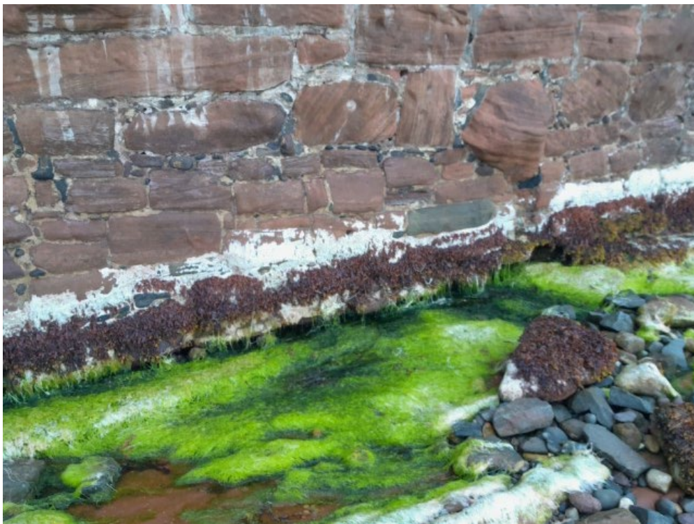
Photograph 15 - Section 3 - 9M 1344Y - Undermining at toe - 18.06.23
