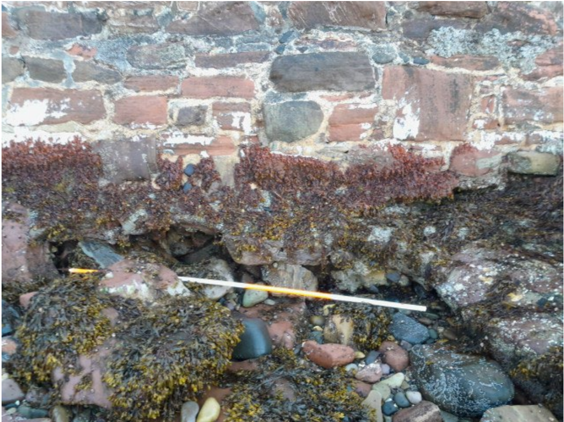
Photograph 20 - Section 3 - 9M 1400Y to 1412Y - Undermining at toe slight det - 18.06.23
