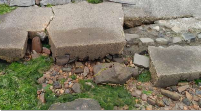
Section 1 - 18M 669Y-Pipe culvert (buried), cracking deterioration blocked
