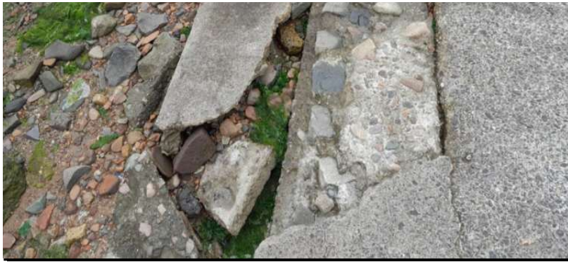
Key 4 - : Section 1 - 18M 0668Y - Washout of concrete haunch along toe -
