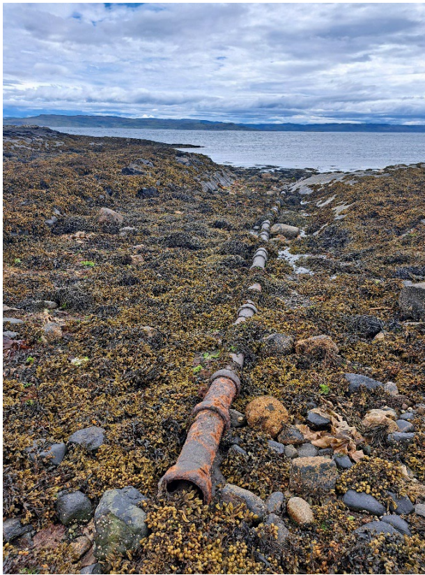
Figure 2 – Cable with split pipe protection on lower shore
