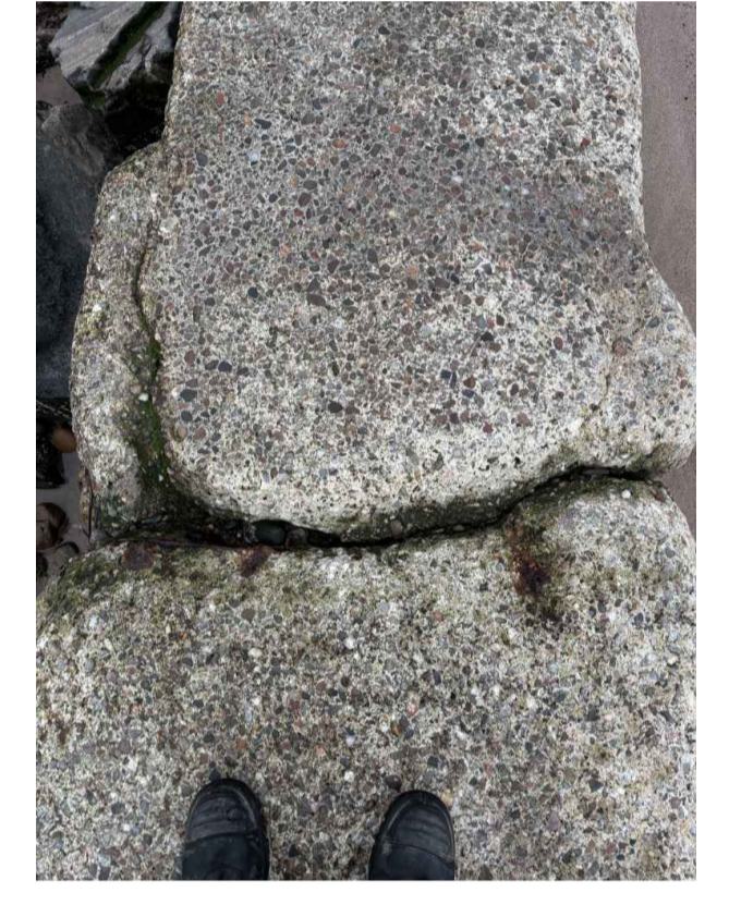
PHOTO 9 COMPROMISED COLD JOINT IN CONCRETE ENCASURE
