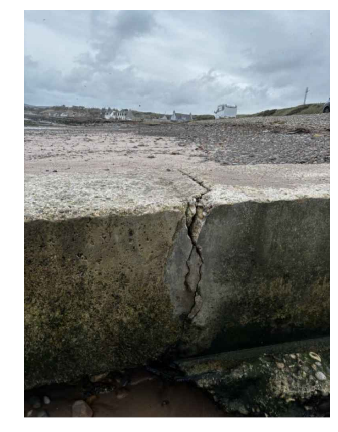
PHOTO 4 DETERIORATION OF CONCRETE ENCASURE AT COLD JOINT
