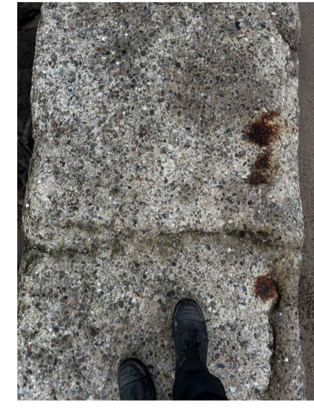
PHOTO 8 COLD JOINT IN CONCRETE ENCASURE
