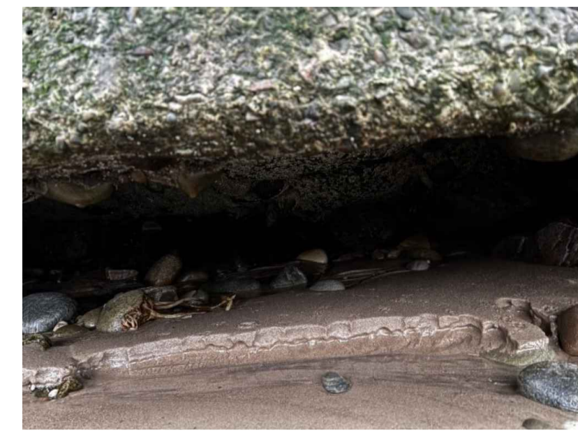
PHOTO 16 EXAMPLE OF LOCALISED LOSS OF BEARING TO UNDERSIDE OF CONCRETE ENCASURE
