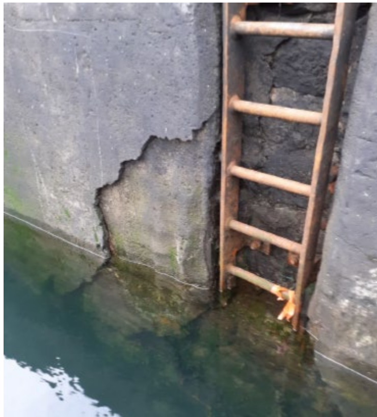
Photo 6 – General view of quay wall showing typical concrete defects
