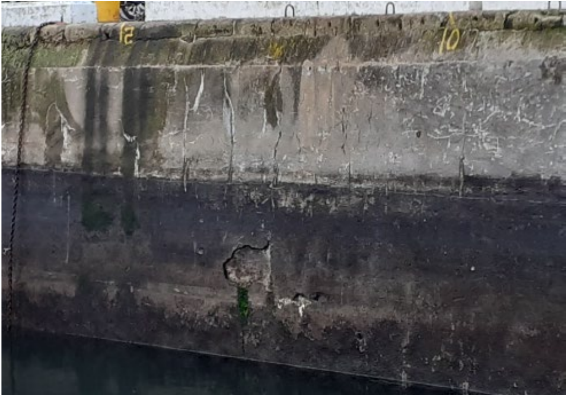
Photo 5 – General view of quay wall showing typical concrete defects
