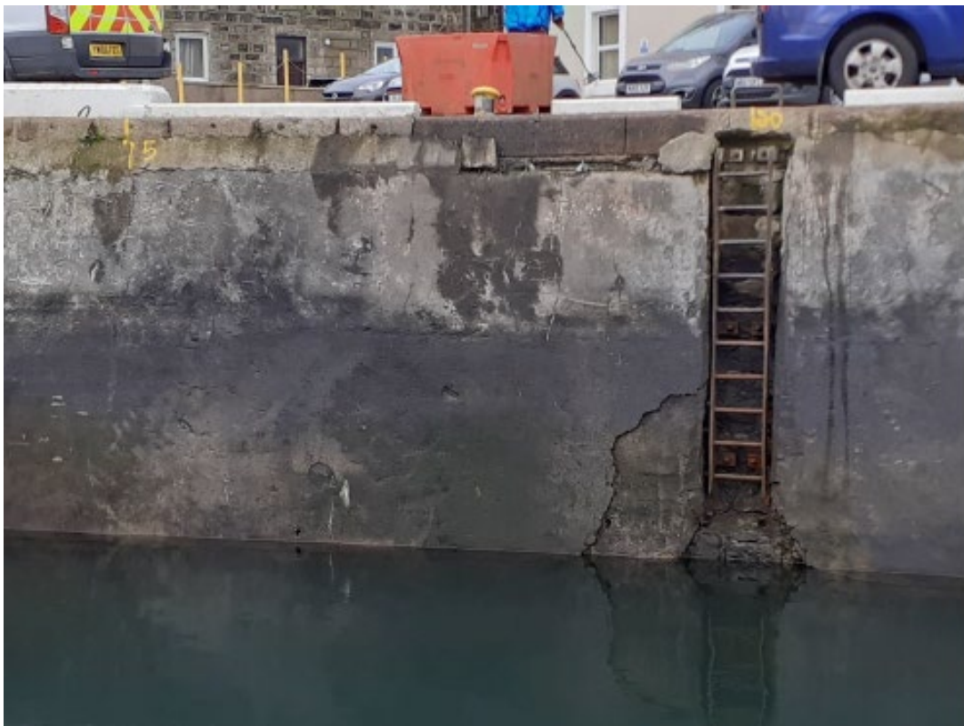
Photo 4 – General view of quay wall showing typical concrete defects and ladder to be removed
